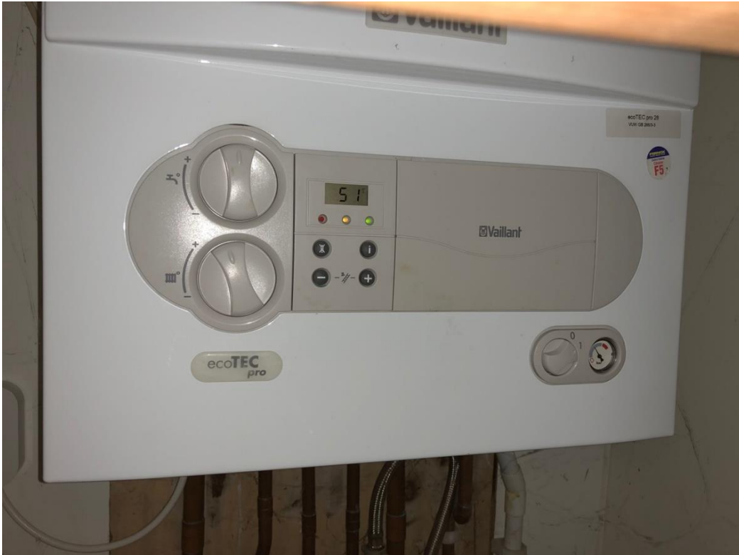
Image 4. Condensing combination boiler, located in the front bedroom. Make and model are clearly identifiable toward the bottom left hand corner of the photograph, and the model 'qualifier' (the specific model type) is visible on the sticker toward the top right hand corner of the photograph
