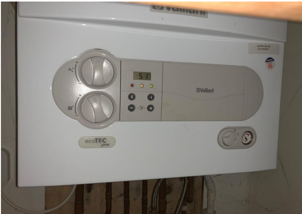
Image 8. Condensing combination boiler, located in the front bedroom. Make and model are clearly identifiable toward the bottom left hand corner of the photograph, and the model 'qualifier' (the specific model type) is visible on the sticker toward the top right hand corner of the photograph
