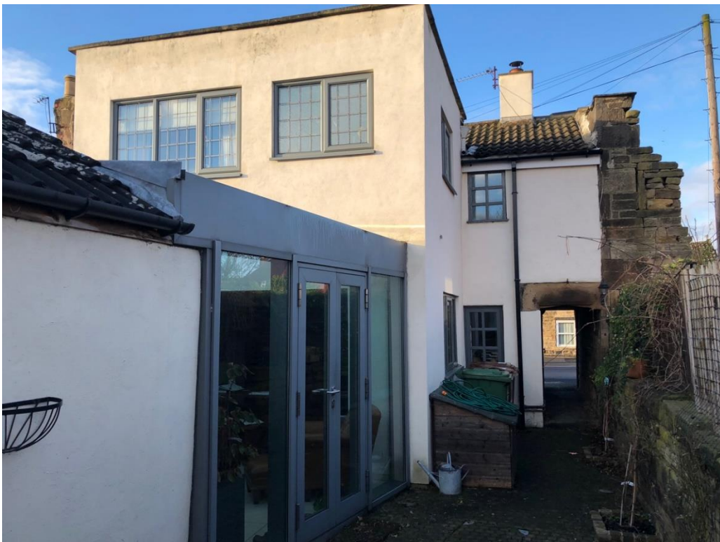
Image 2. Rear elevation of control property for phase 1 of the EPC study, showing two storey circa 1970 extension, and glazed kitchen extension beyond this. The building that adjoins the kitchen extension to the left hand side of this photograph belongs to the neighbouring property.
