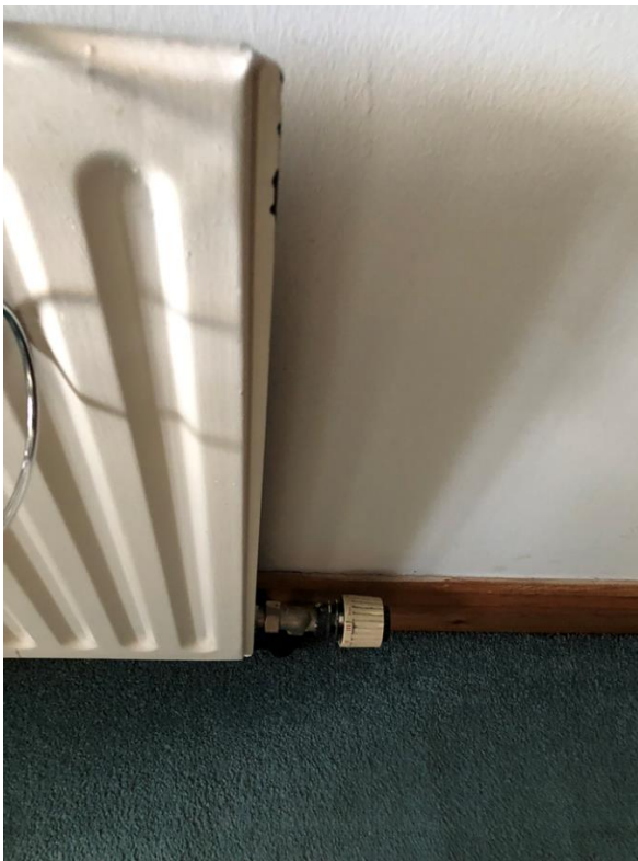
Image 10. Thermostatic radiator valves, or 'TRVs' are common. These allow the temperature of individual rooms to be adjusted, while the smart thermostat will control the overall temperature of the dwelling from its central location.
