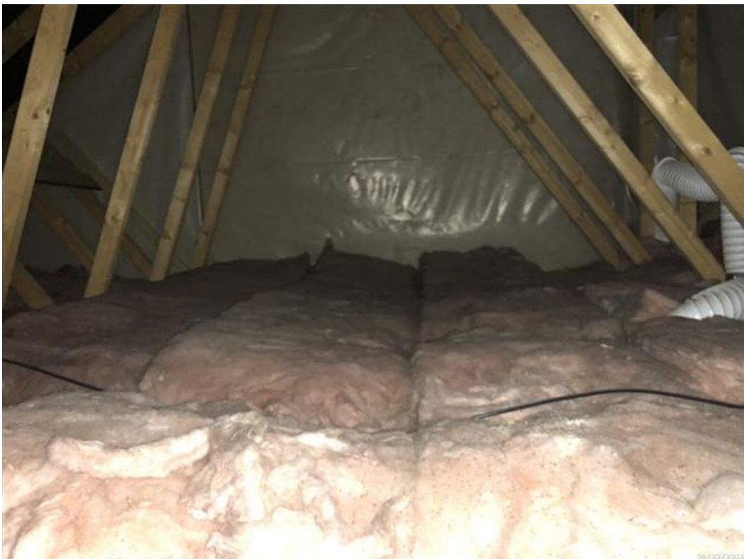
Image 3. A wider view of the loft insulation, showing a consistent, relatively even level throughout. Note also here the view of the party wall, with the grey plastic sheet over it. It can be hard to identify the
