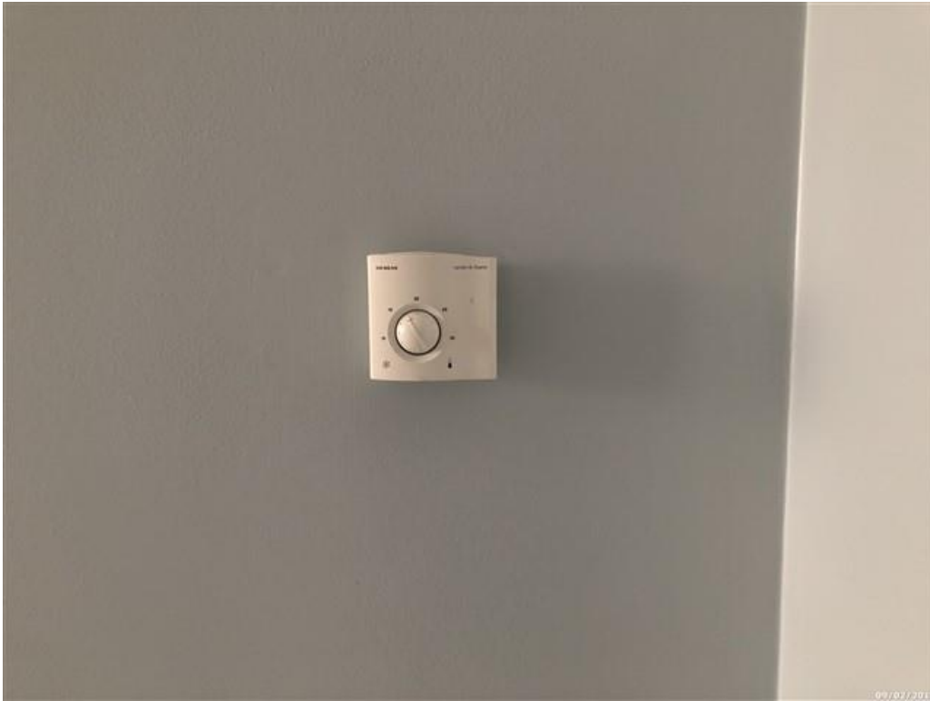
Image 10. A traditional wall mounted thermostat, fitted in the property on construction in 2000.
