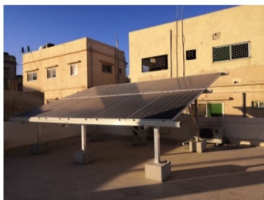
Figure 1. The PV installed at the house, Jordan.
