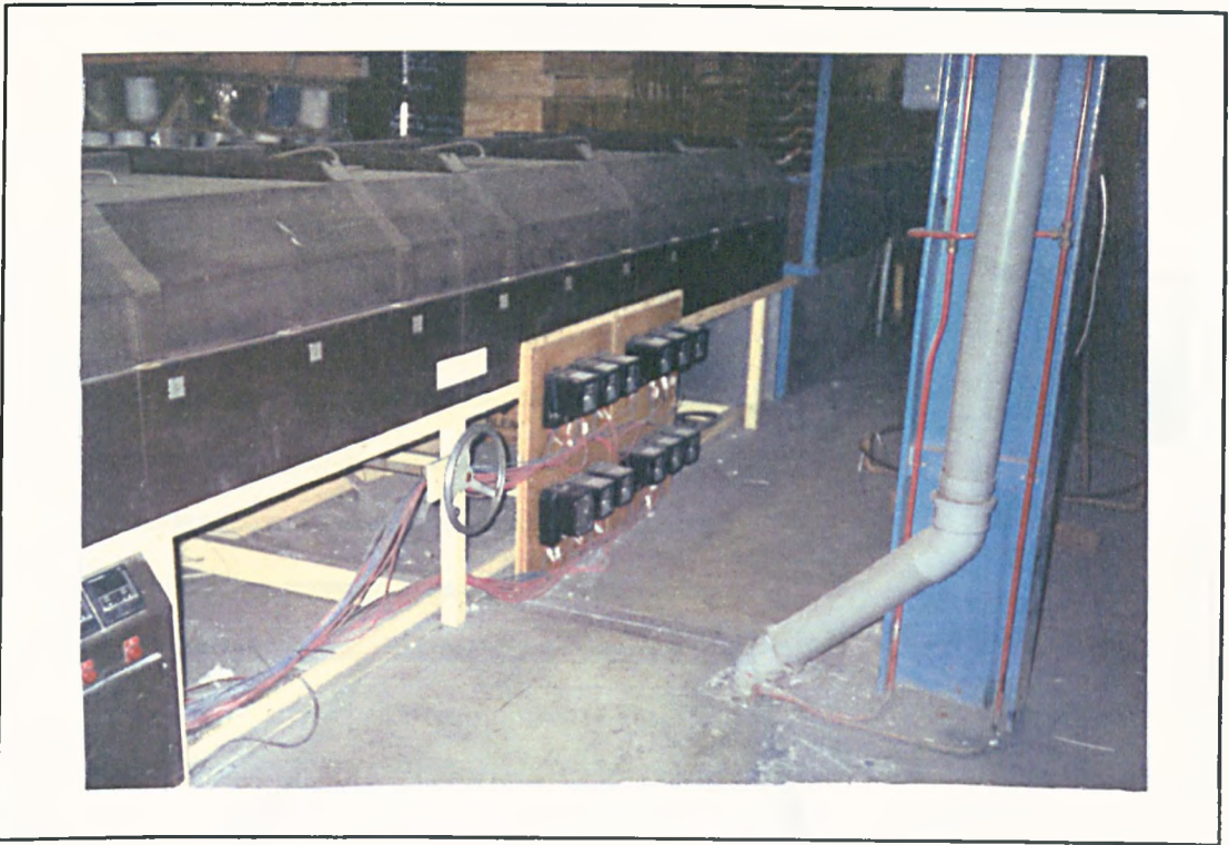
Figure 3-3. Photograph showing the Kilowatt-hour meters installed on the Furnace.
