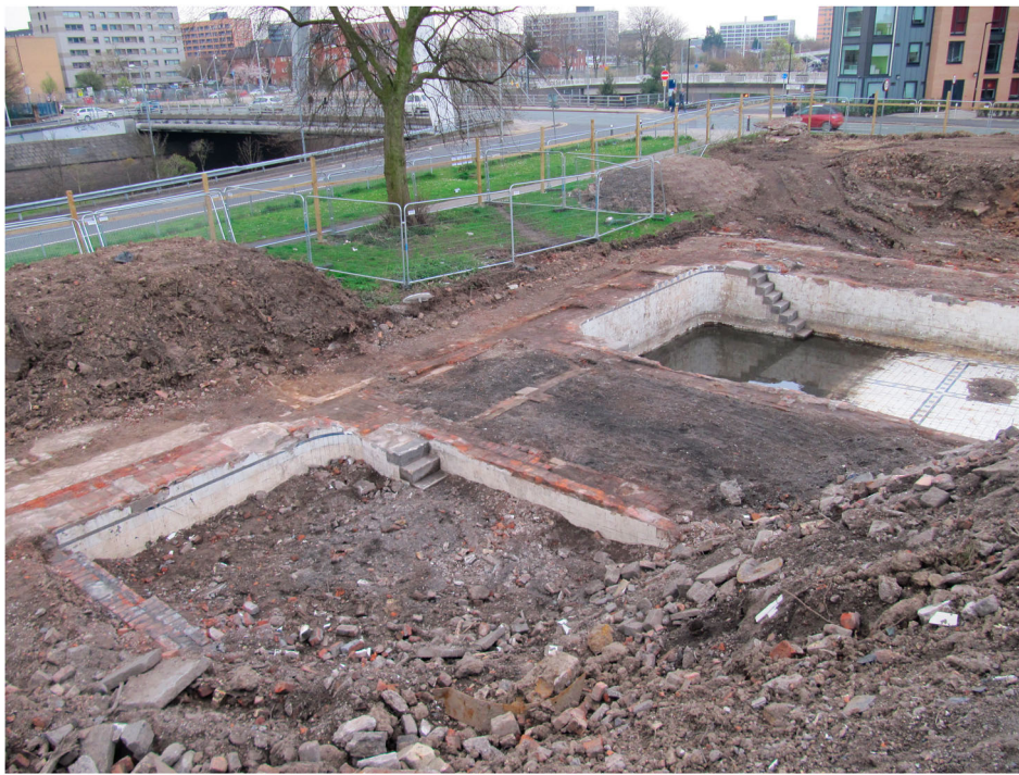
Figure 17. Leaf Street Baths during excavation, showing the second-class pool in the foreground and the first-class pool to the rear (© University of Salford).
