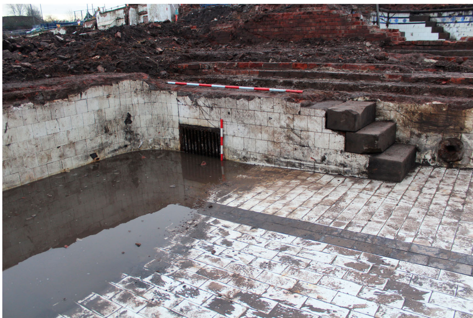
Figure 12. The cast-iron grate across the drain and the collared pipe associated with the filtration system in the second-class pool (© University of Salford).
