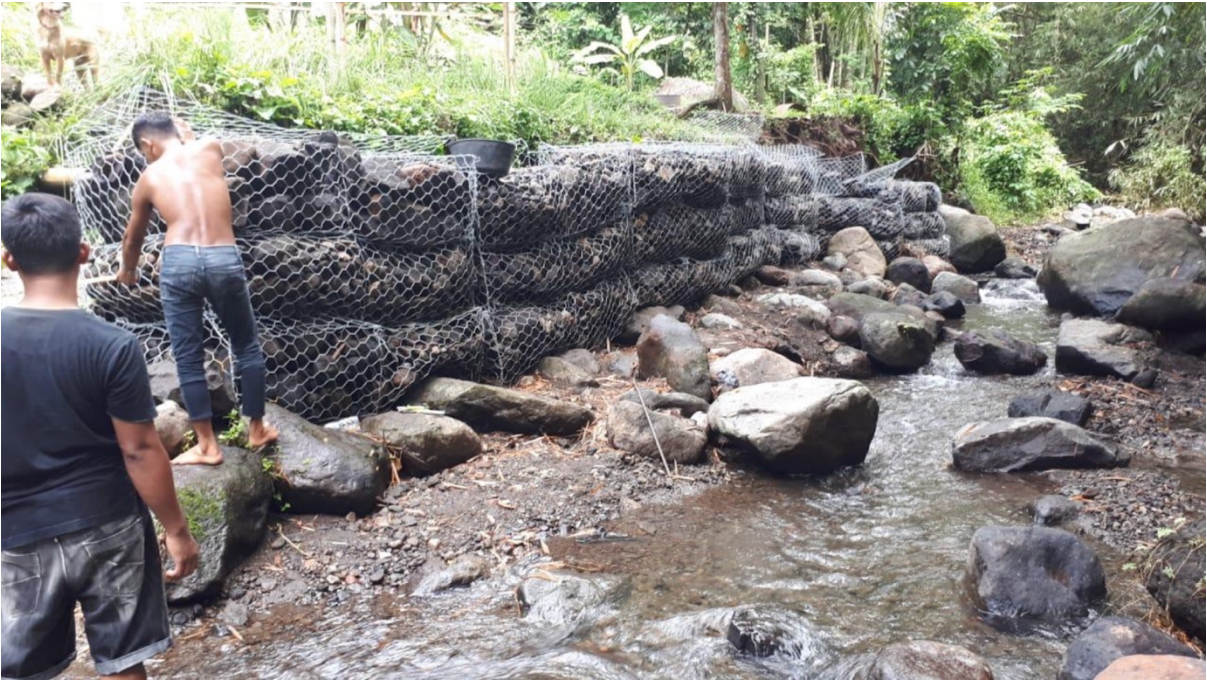
Figure 21: 40-meter riverbank gabion basket retaining wall. Source: Omah Lor owner
