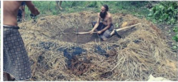
2 layers of soil, Biochar and straw build the banks of the pit
