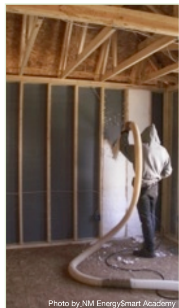
Photo by NM EnergySmart Academy
