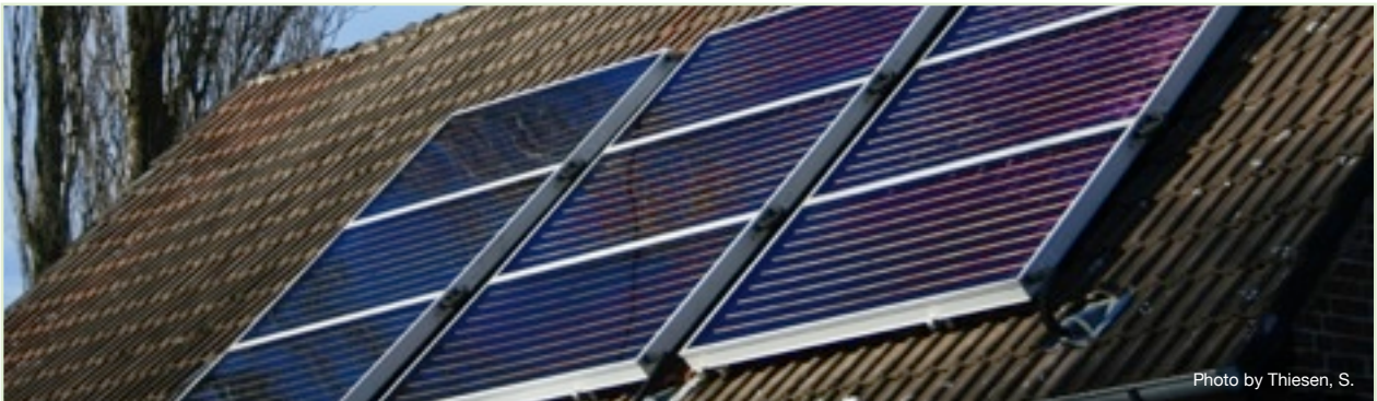
These collectors provide heating for a 1500 litre water tank and space heating system
