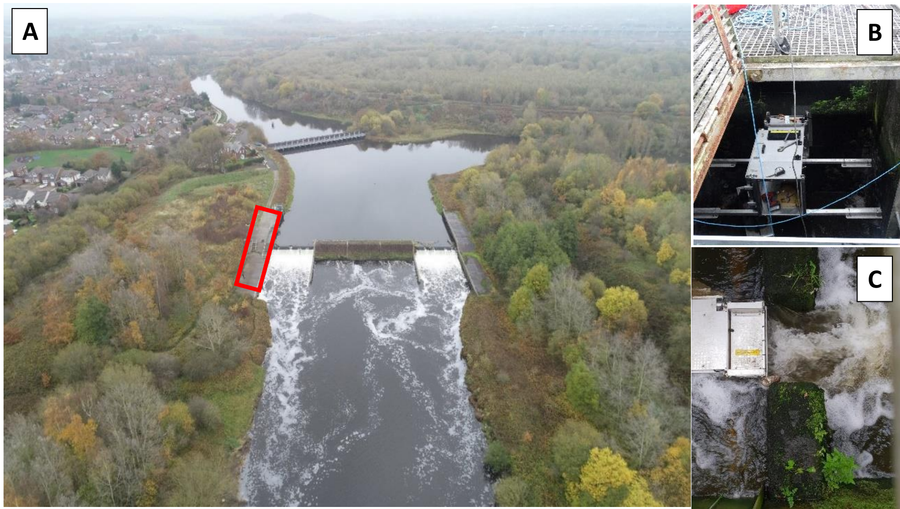
Figure 5: a) Drone image of Woolston weir (courtesy of Dr Neil Entwistle) with the fish pass where the Vaki River-watcher has been installed (highlighted in red); b) Vaki River-watcher being installed in the weir; c) Installed and working Vaki River-watcher.
