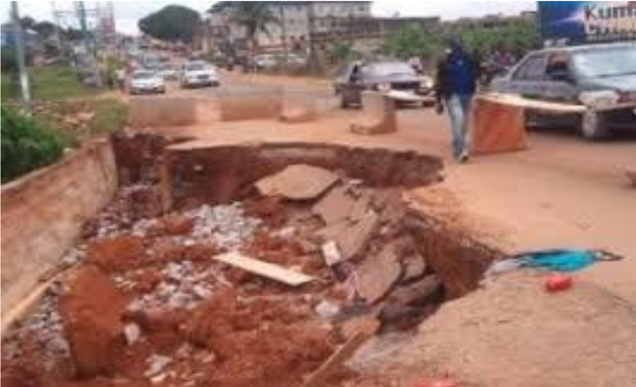
Appendix H: Annotated of the condition of some Ghana roads
