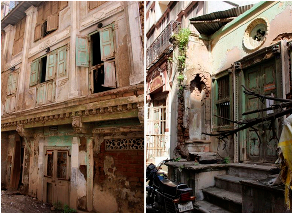
Figure 6. Dilapidated heritage buildings in need of restoration in Rander Gamtal (Source: authors' photos).
