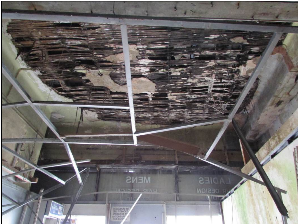
Plate 6: The interior of the main room, showing the exposed lath and plaster ceiling
