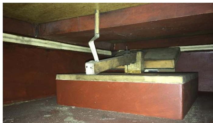
Photograph 5 Internal control valve
