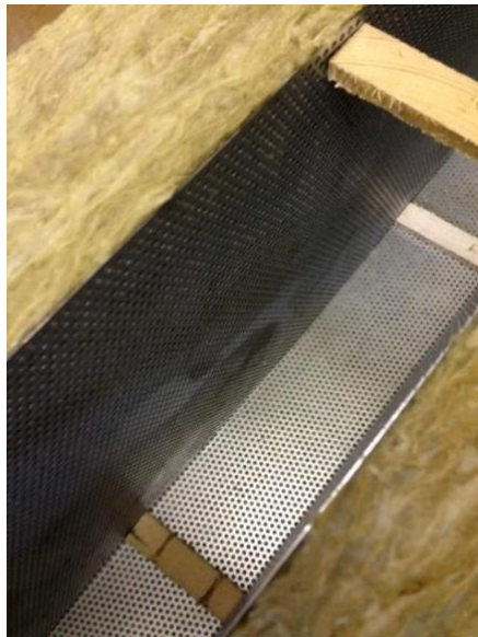
Photograph 35 Duct silencer with 100mm mineral wool and perforated metal lining
