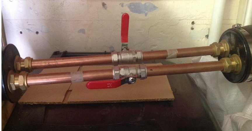
Photograph 27 Two isolating gate valves
