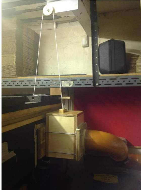
Photograph 25 External Roller-blind valve
