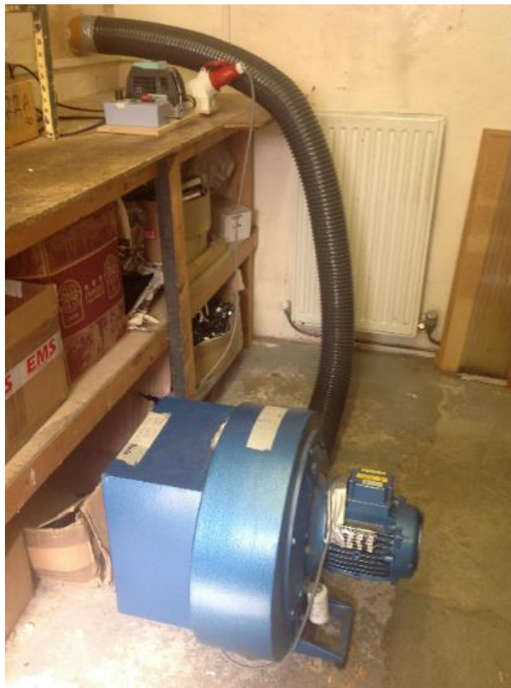
Photograph 3 3000 rpm blower with flexible connecting pipe
