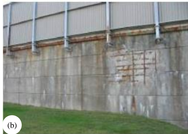
Figure 2.3: General corrosion of steel in concrete (a) underside of bridge deck and (b) Retaining wall of bridge (Hansson et al., 2012)
