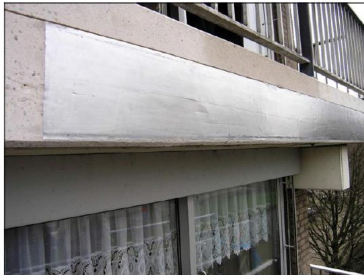
Figure 2.28: Zinc sheet anode applied to a concrete balcony, prior to overpainting, (Broomfield, 2000)
