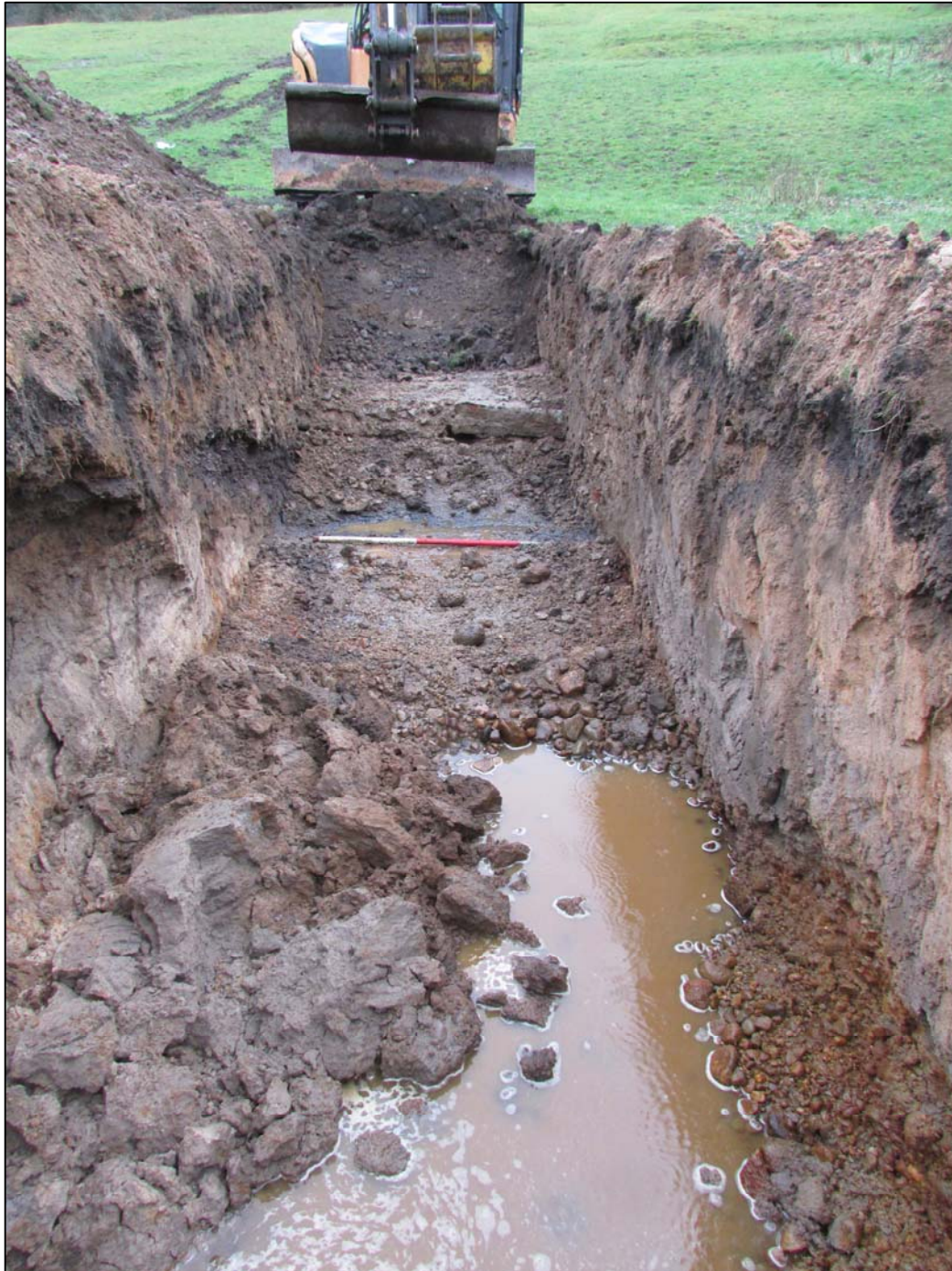
Figure 10: Detail of the western end of T1 looking at the cut and silt marking the line of the leat.
