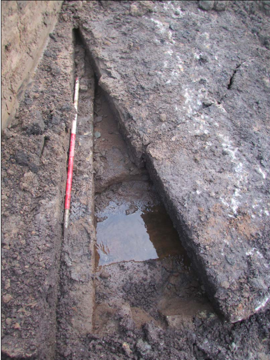
Figure 19: T3 looking at the silts and water within the culvert.
