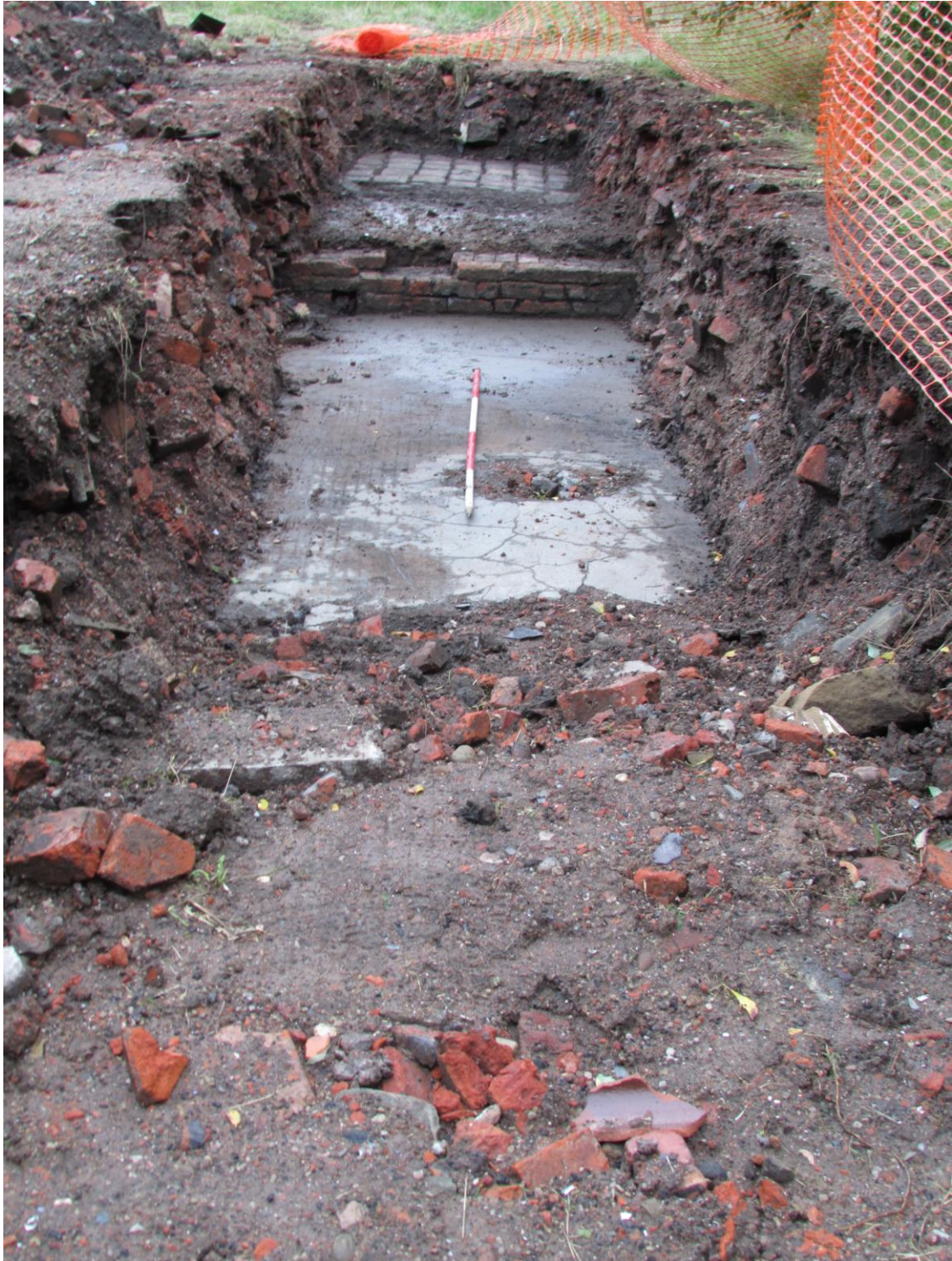
Figure 16. Trench 3, showing the concrete floor of the Brass Foundry and outer wall, with the cobbles of Cawdor Street in the back. Looking South
