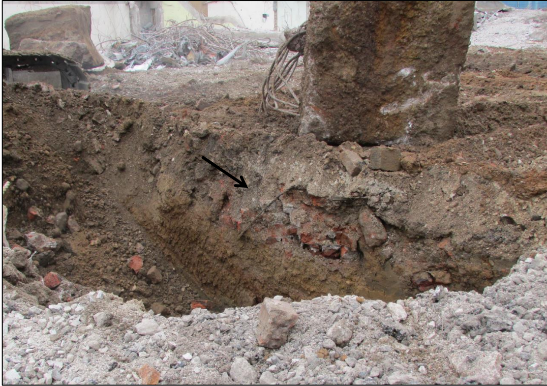
Fig. 7 Walls relating to the Female Misdemeanant Wing still survive (as shown above), however they were frequently shallow and the natural geology is visible here at 0.50m below the surface
