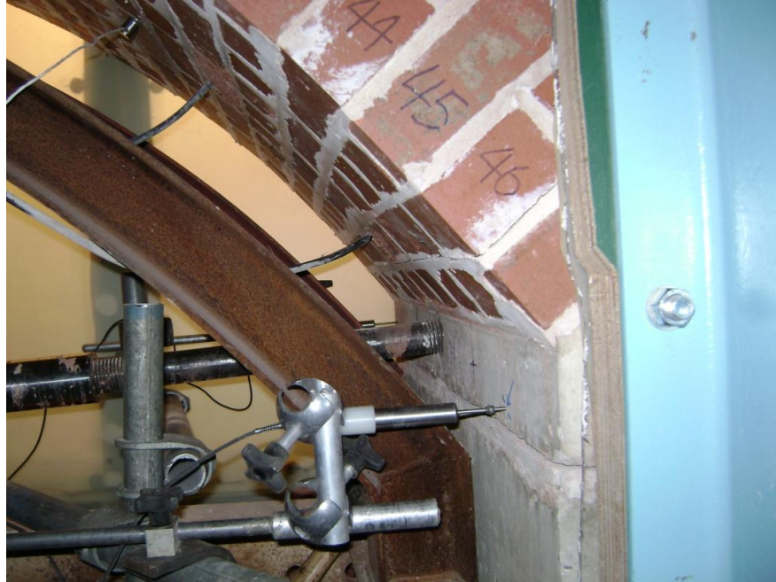
Figure 2.22 – LVDT displacement gauges positioned on skewback and soil pressure cell data cables passing through arch intrados to data acquisition system
