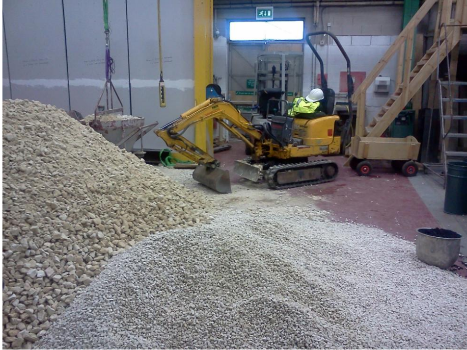
Figure 2.16 – Fill material, main fill MOT type 1 limestone (left) and course fill for PIV (bottom)
