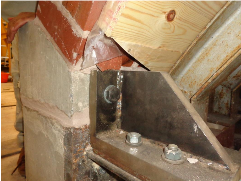
Figure 2.11 – Fixture of tie beam to lower abutment and removable upper restraint to skewback
