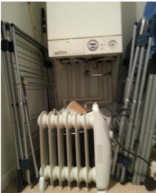
Figure 3: Electric convector heater stored in cupboard. Note also the boiler is older and does not have a qualifier available as per Figure 1
