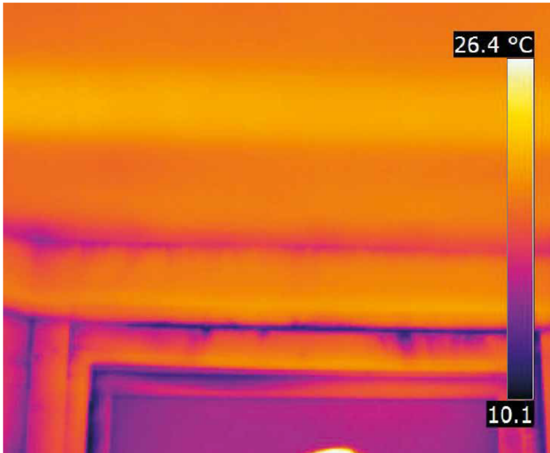
Figure 4. The cold air entering around the window edges is clearly visible using the thermal camera.
