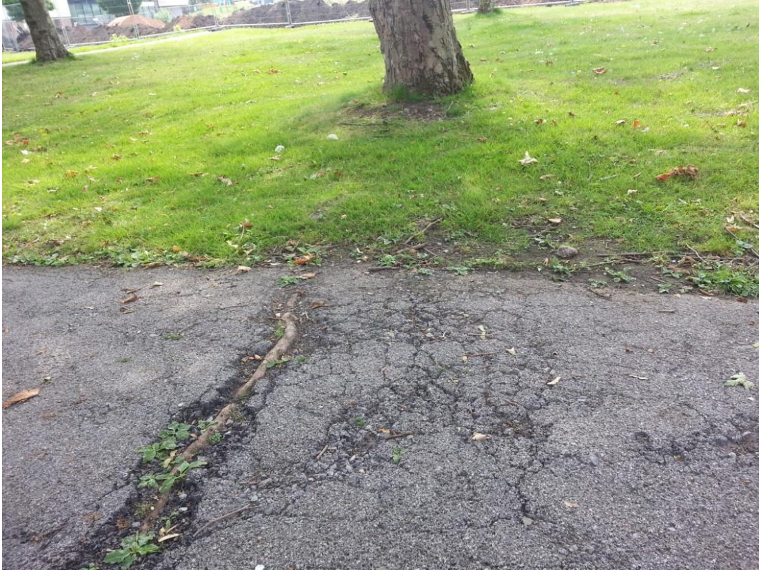
Fig. 6.7: Some examples of tree roots damage to impermeable pavements of Site 2. Photos were taken by Vincent Uzomah.
