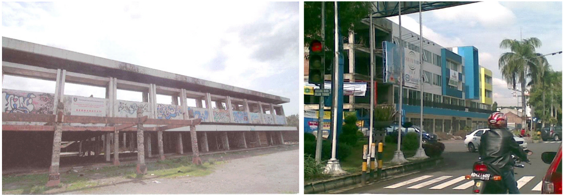
Figure 5.4. (a) Ex 'Super Ekonomi' Shopping Centre after the conflict, recently was built into (b) Solo Centre Point in 2011
