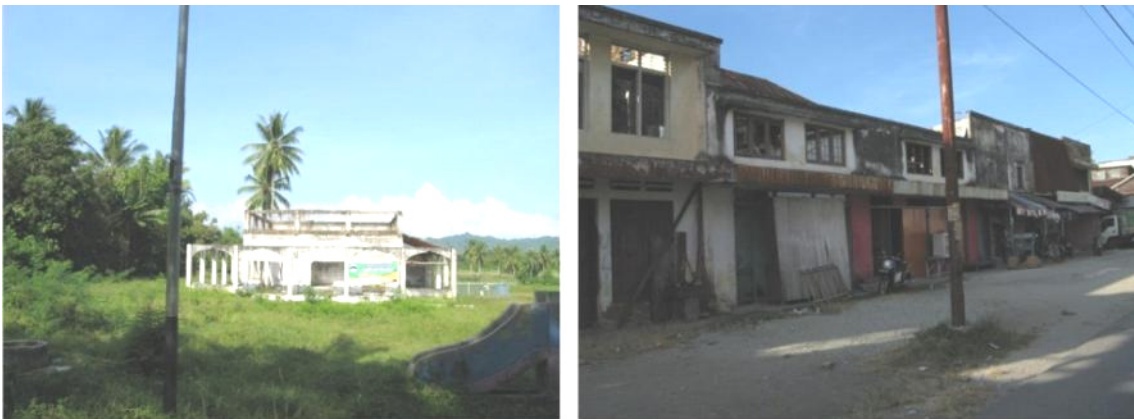
Figure 5.14. Ex traditional religious boarding school; (b) burnt houses along previously vibrant street remains the same until 2011 Source: Field observation, taken in November, 2011.
