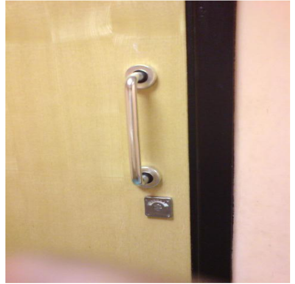
Figure 8 Same door with metal handle on the other side
