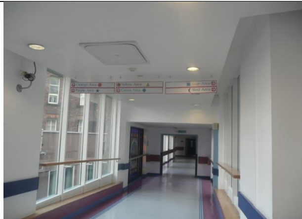
57: However, the sudden appearance of blue on the skirting boards here communicates a different message. One starts to wonder at this stage whether the purple colour is intended to lead the user to the purple zone or purely for decorative purposes.
