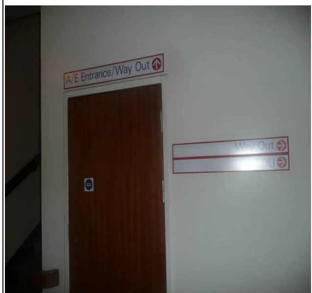
33: Is it though the door, up the stairs or to the right? As it happens, the door seen here is a cupboard and just at the top of the stairs is the symbol for no unauthorised entry (see pic 10). Could it be the case that this symbol was put to clear this confusion?
