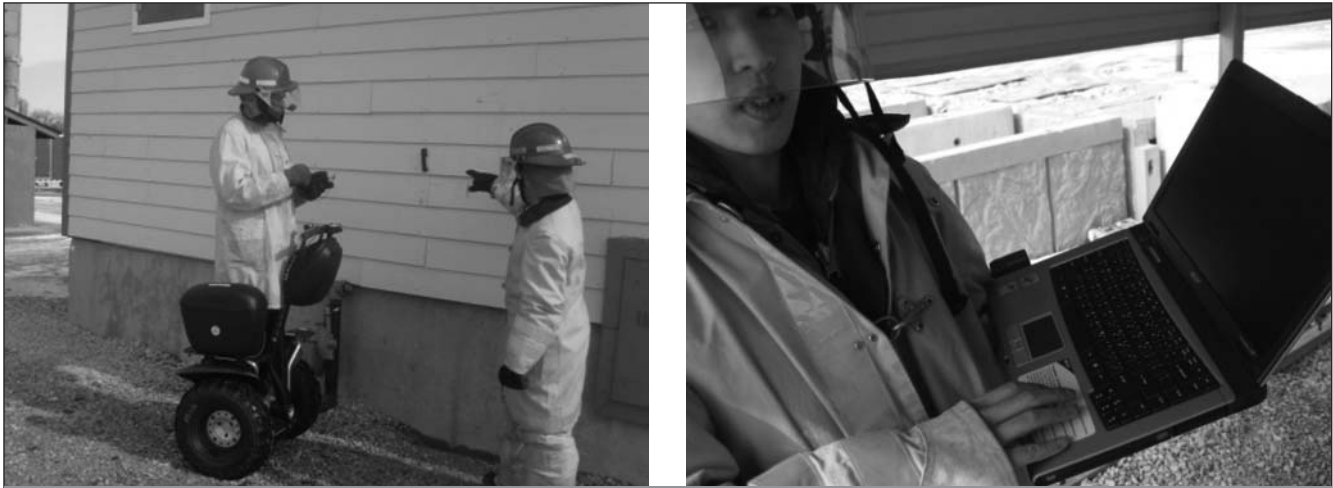
Fig. 12. Recording building assessment information (a) using RFID tags and (b) accessing Web-GIS system using telecom network
