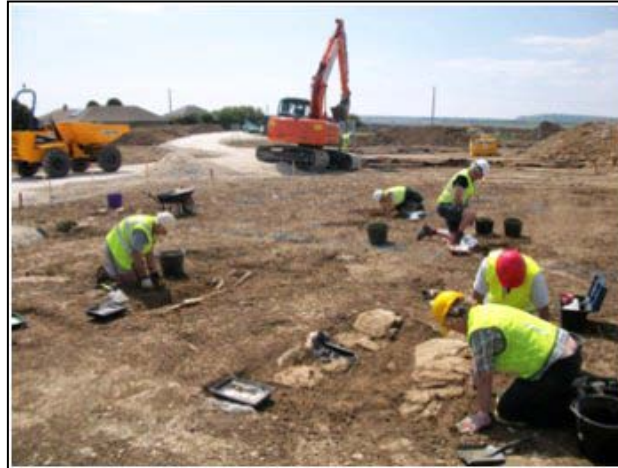
Volunteer archaeologists excavating a graveyard found on the edge of the development (©WCPT)
