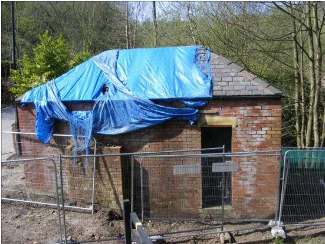
Fig 1: The 1920s substation at Park Bridge supplied the Ironworks with lighting and power.
