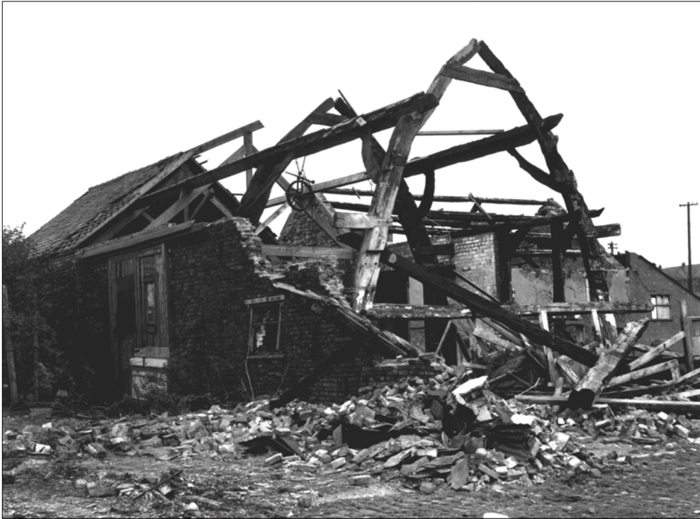
Plate 1 – Newton Hall in 1969 prior to restoration, showing the 18 th century threshing barn during demolition
