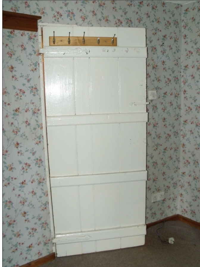
Fig 6: The plank and baton door on iron gudgeons and with iron strap hinges in FF4.
