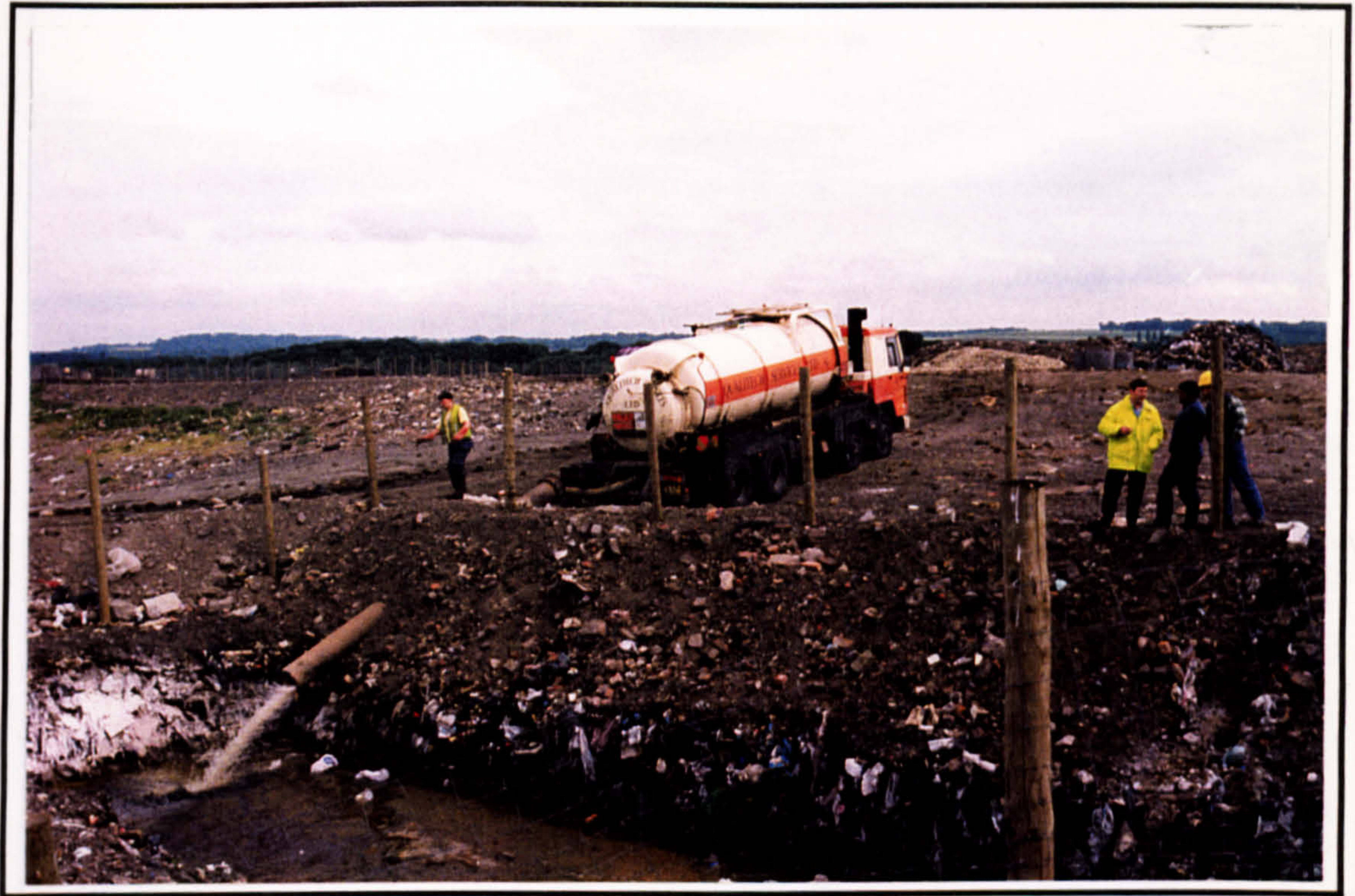
Plate 1-13: Sludge or liquid wastes is drained into the pits
