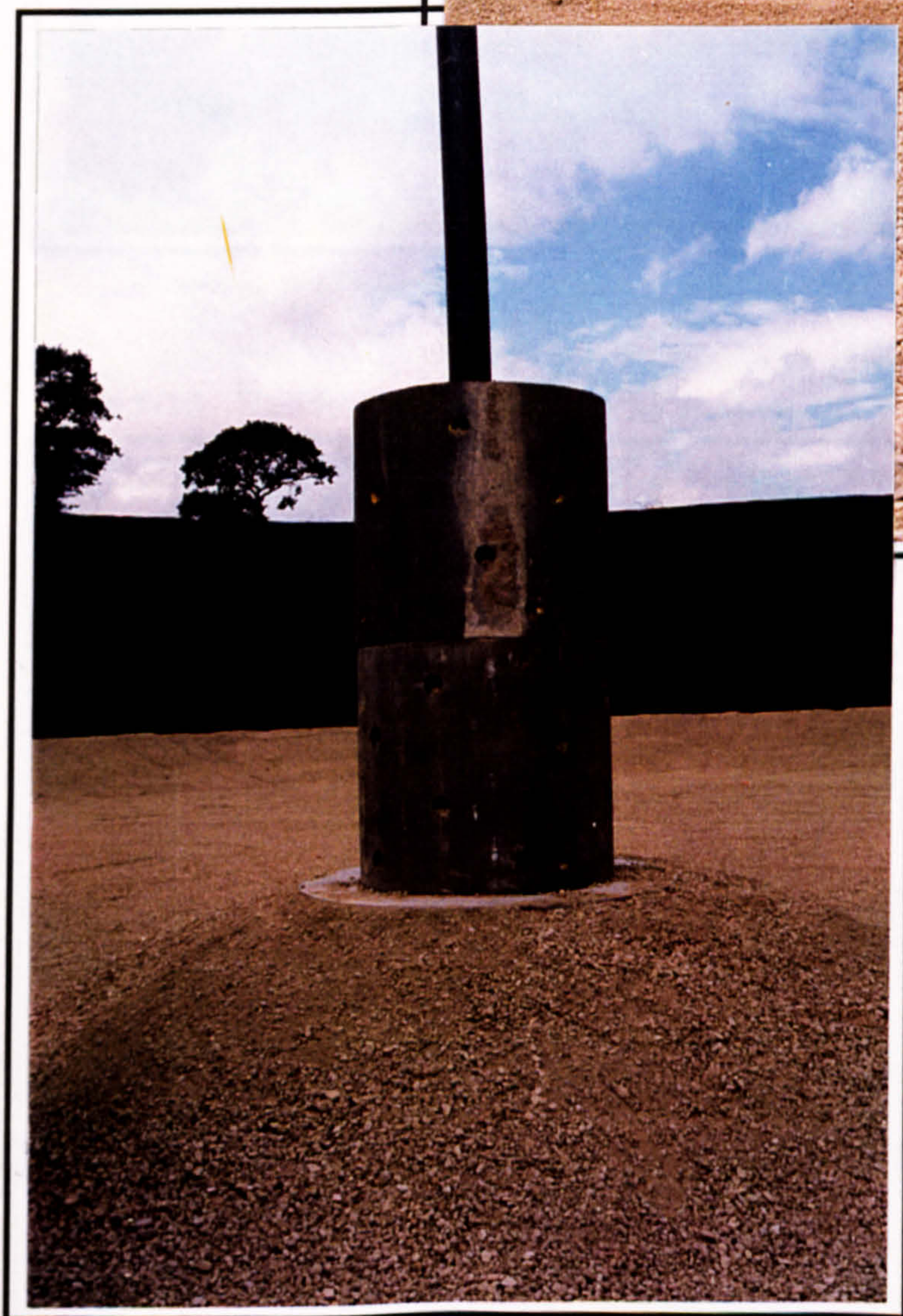
Plate 1-8: Leachate monitoring well
