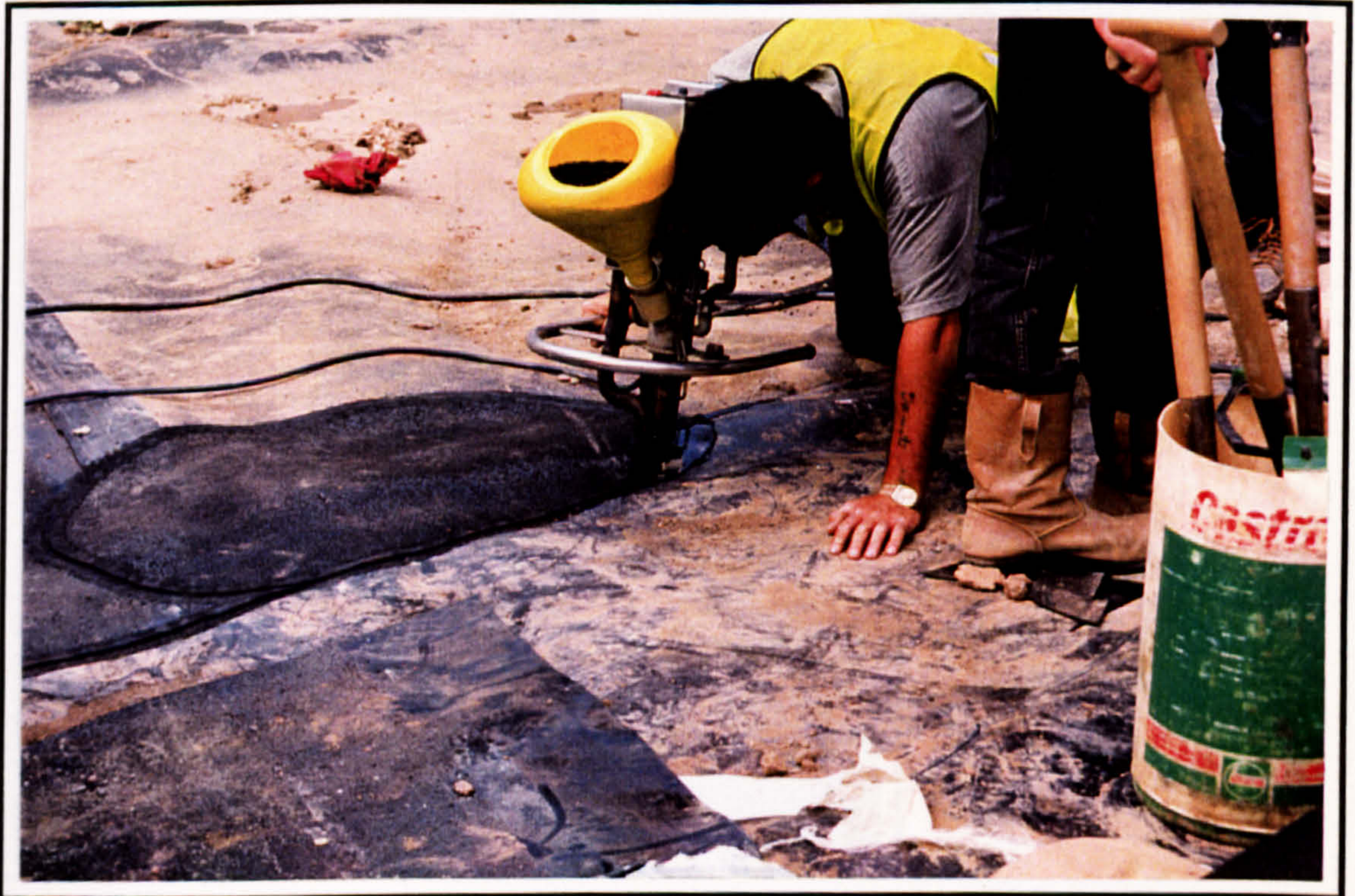
Plate 1-6: Joining the HDPE liners after the wire is properly sealed around the joints
