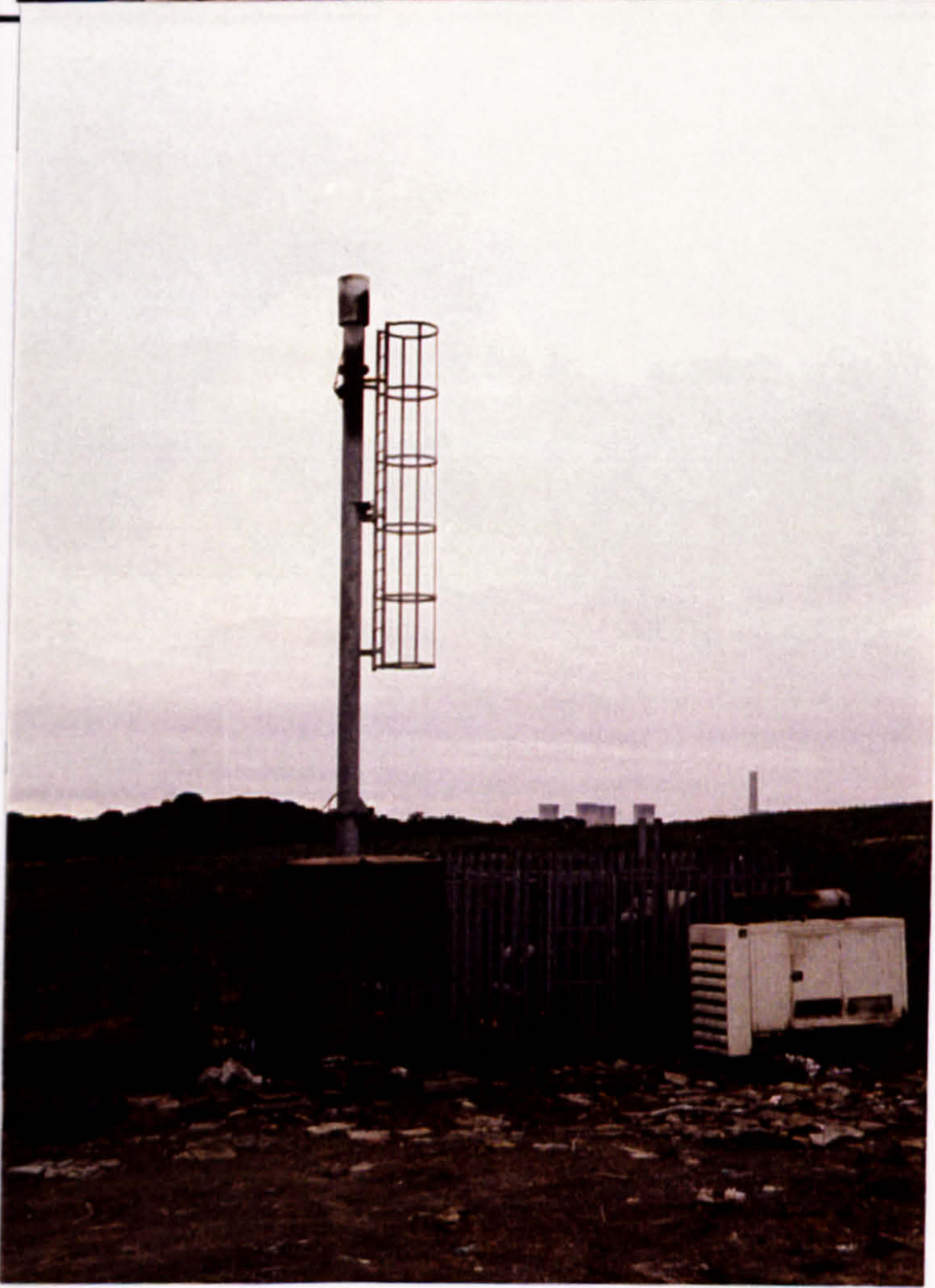
Plate 1-18: Flaring of methane gas and methane pump station
