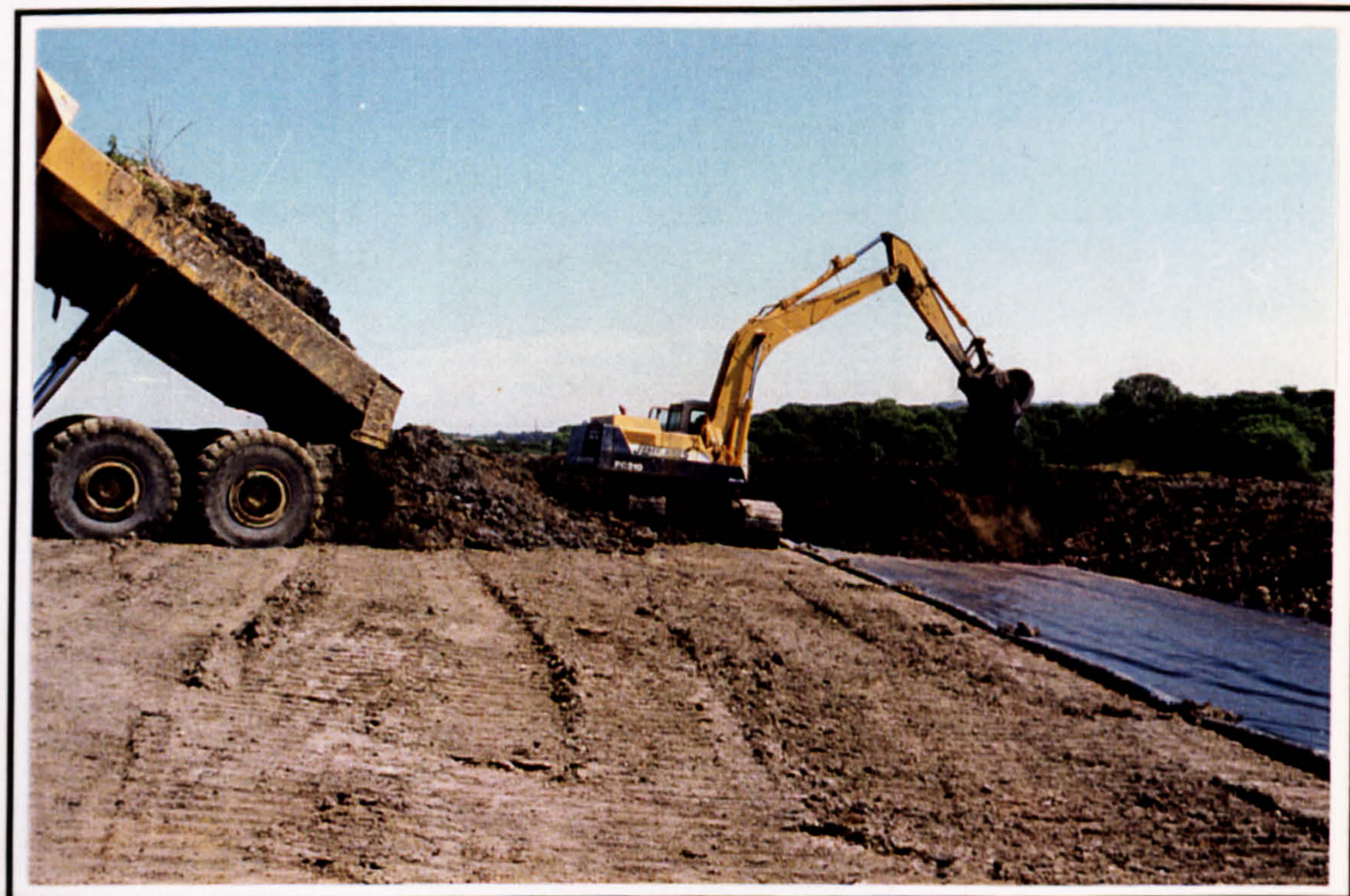
Plate 1-16: Recapping of the wastes with the HDPE liner and the top soil
