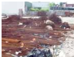
Figure 17: The Disorder Caused by the RC Steel Piles Due to Contract Constraints
