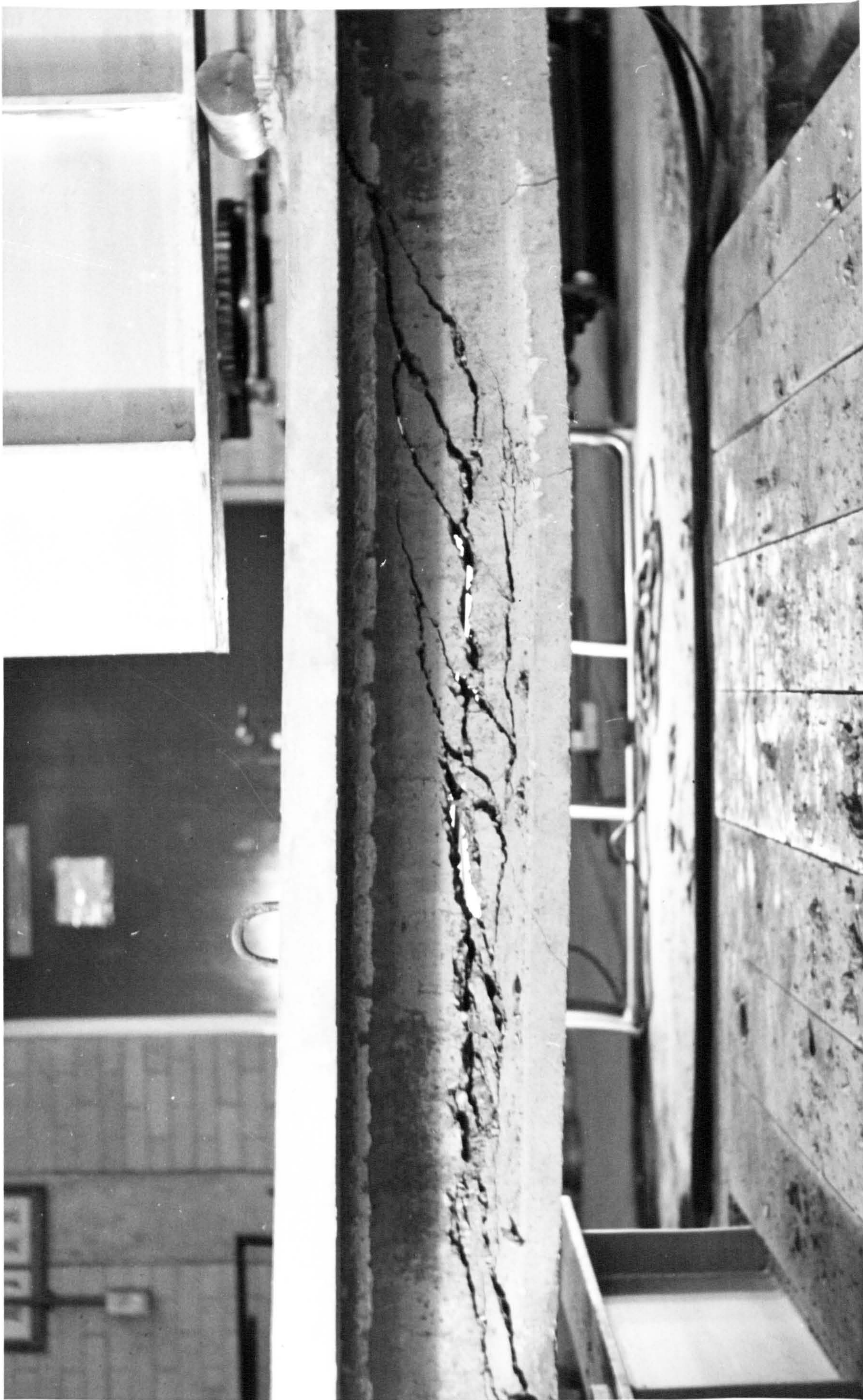
PLATE 5.2. - SHEAR FAILURE - SERIES X
