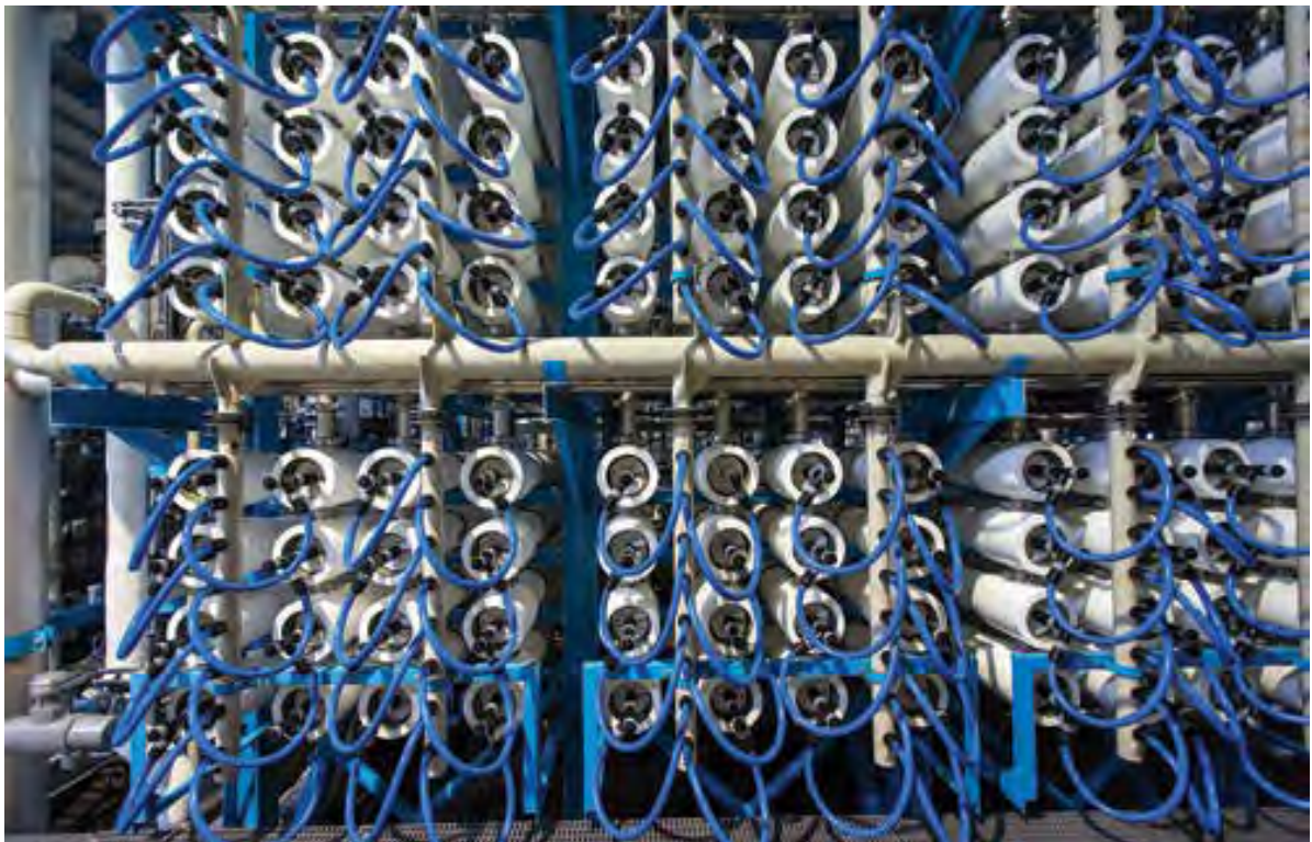
Figure 5-5. Pressure vessels connected in parallel in CDP. Courtesy WaterWorld 2018.
