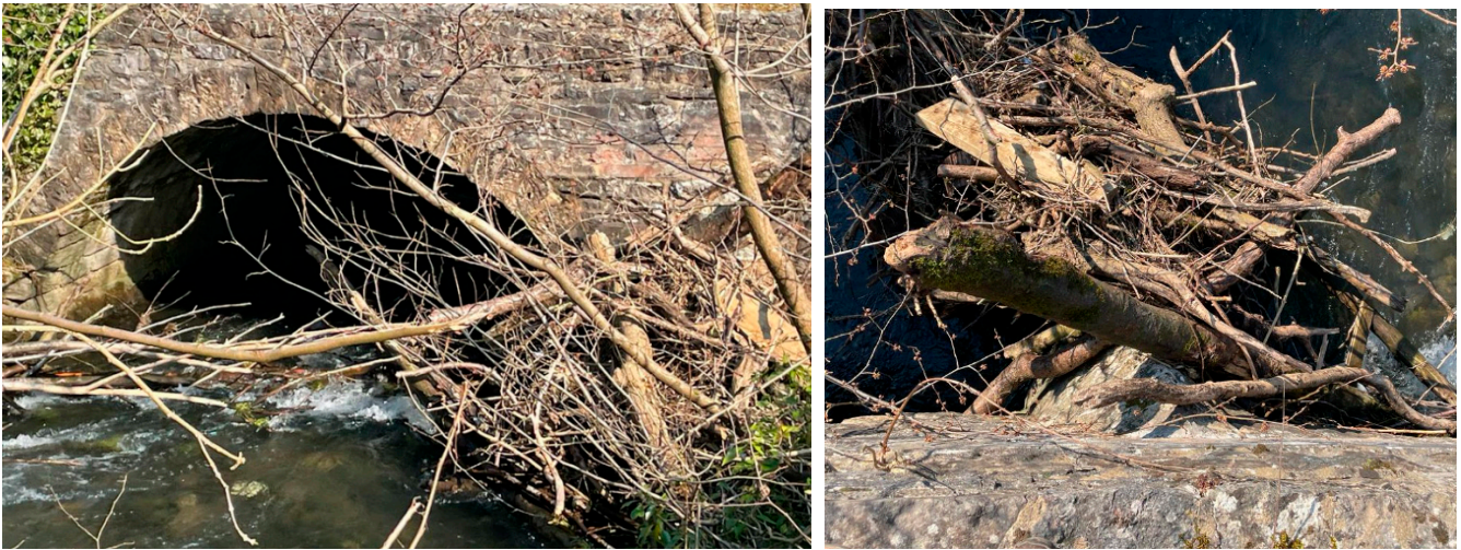
Figure 2. Debris accumulation at the bridge cutwater (the streamlined head of the bridge pier) in the River Wye in Derbyshire, UK (Image by Eda Majtan).
