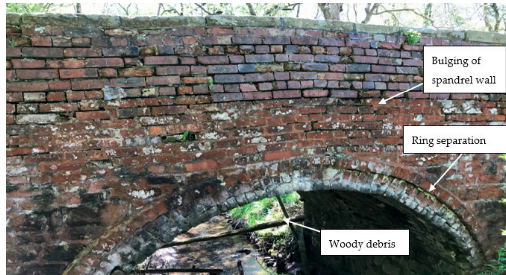
Figure 1. Downstream elevation of a single-span brickwork arch bridge spanning Bollinhurst Brook in Lyme Park, Cheshire, UK, with woody debris located upstream and damage at the spandrel wall and arch barrel (image by Eda Majtan).
