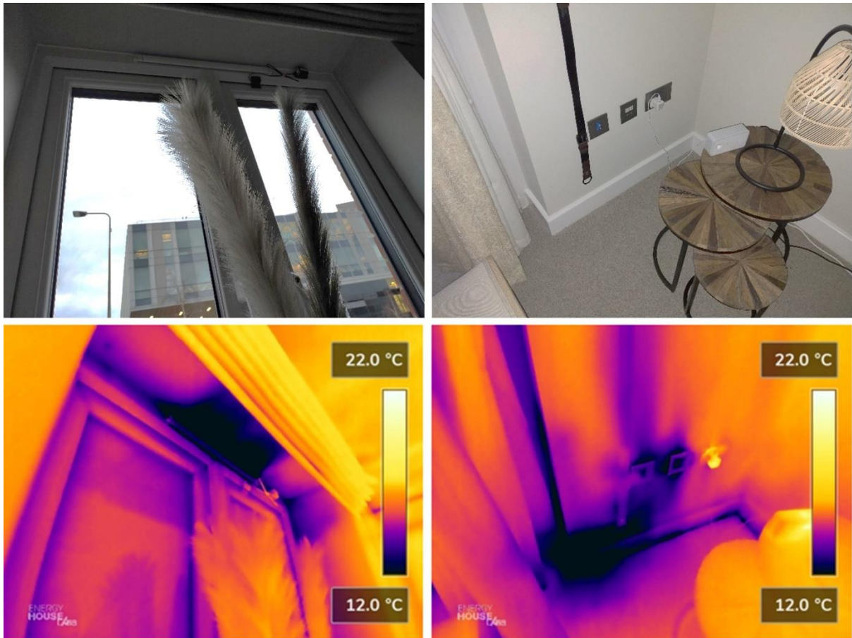
Figure 4.13 Air infiltration was observed through closed trickle vents both prior to and during the blower door test (left). Air movement behind the plasterboard around the window and door was also revealed (left and right). Air infiltration into the dwelling from the door was revealed at the ground floor junction and through external wall mounted services via the plasterboard void (right).
