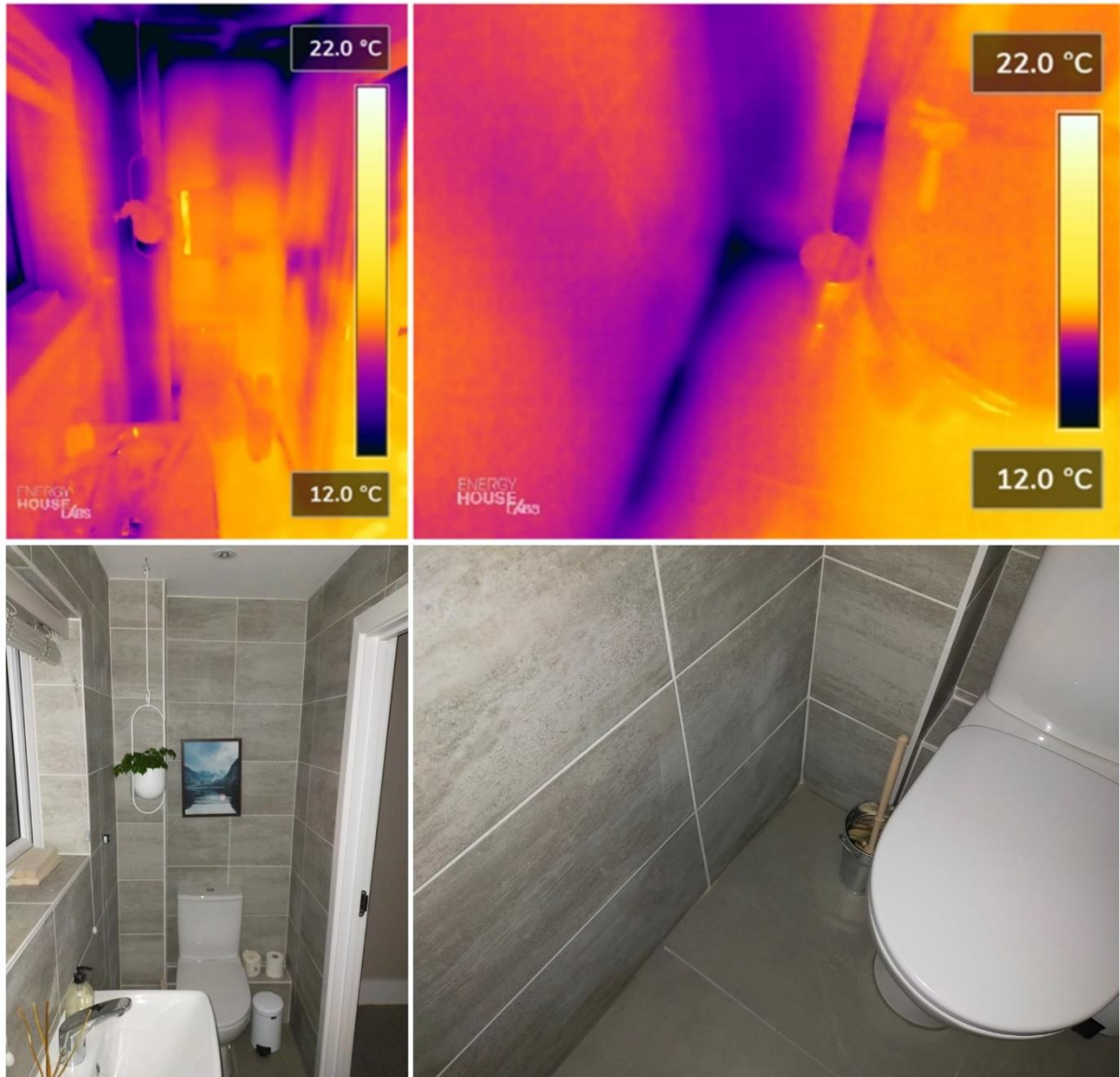
Figure 4.9 Air movement within the SVP void in the first-floor bathroom (left) with some air infiltration evident at the interface between the void and intermediate floor (right)
