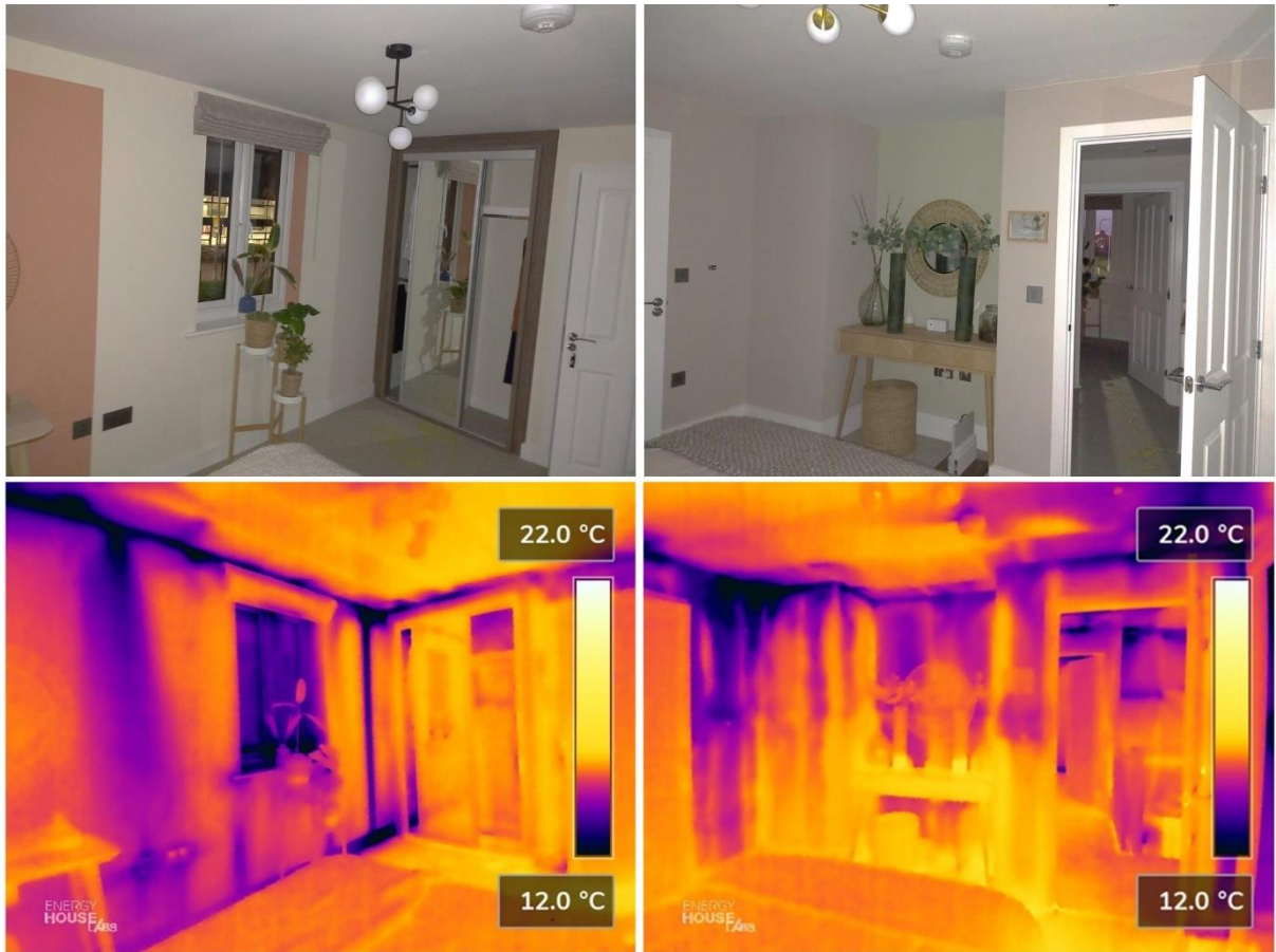
Figure 4.12 Examples of cold air movement from the loft space behind the plasterboard of the external (left) and internal (right) walls
