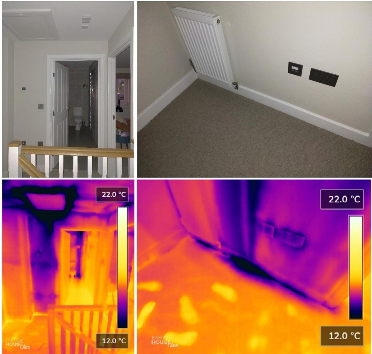
Figure 4.11 Air movement from the cold roof space into the internal partition wall. Air infiltration into the habitable space was evident through the wall mounted services and at the junction with the intermediate floor (left and right). Direct air infiltration was evident around the loft hatch (left).
