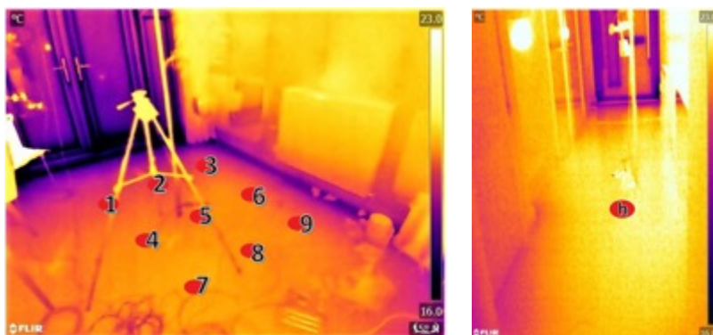
Figure 33. Thermogram showing locations of floor in-situ U-value measurements (a) Kitchen (b) Hall.
