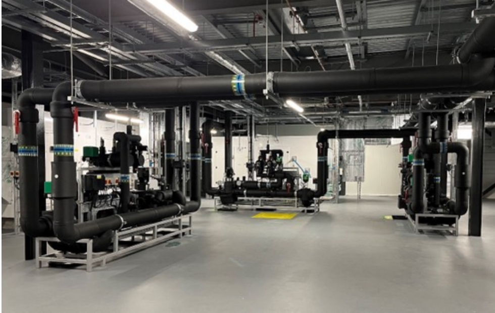
Figure 4. HVAC systems providing close climatic control to chambers
