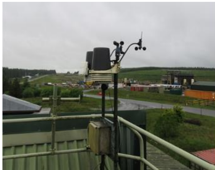
Figure 84 - Automatic Weather station situated at DNV Spadeadam R5BC Control Building.
