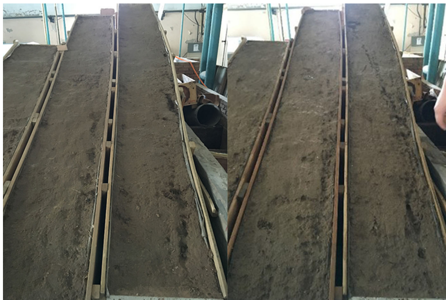
FIGURE 10 Scouring of the lower part of the slope.
