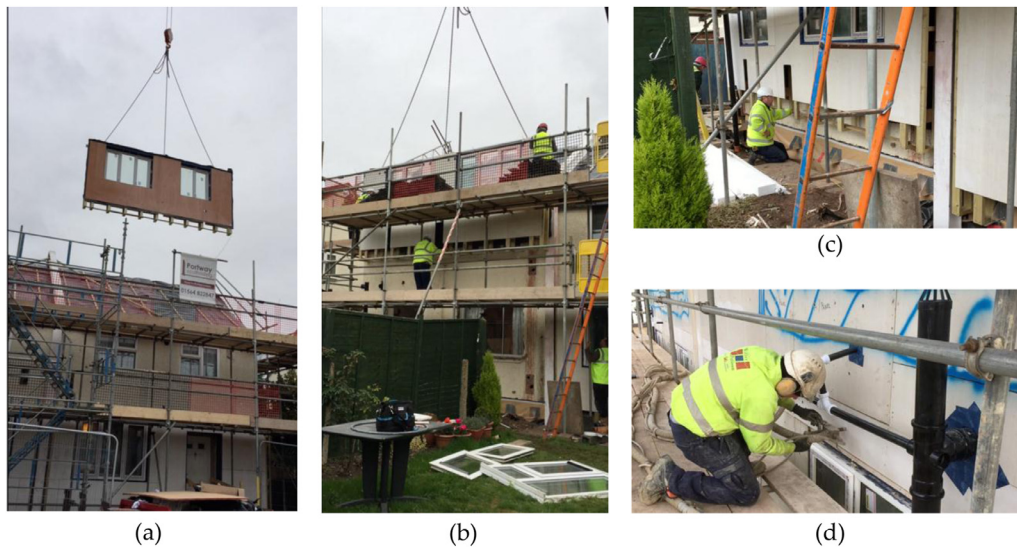
Fig. 8. Installation of the retrofit thermal envelope: (a), (b) and (c) – Stages of installation of an external prefabricated envelope panel; (d) Injection of thermal insulation into the installed external panel (source [7]).
