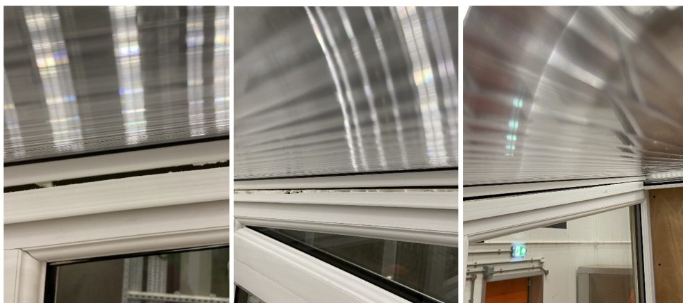
Figure 9 Show Sealant Disparity Across Different Areas of the Ceiling (More Visible During Scenario 2)
