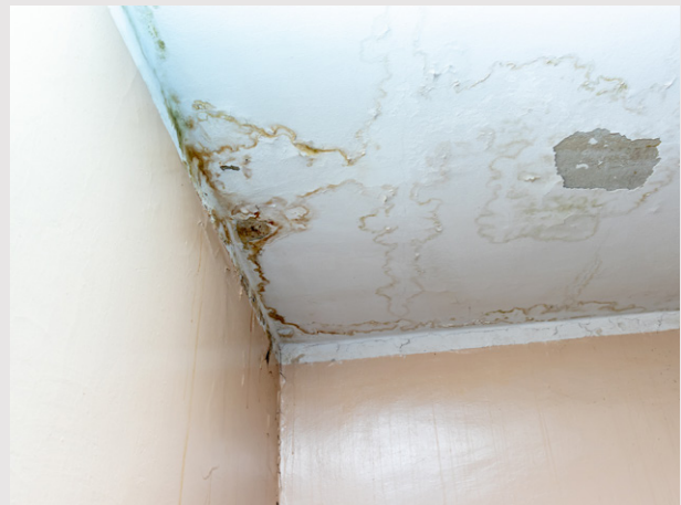
D Stains, rot or mould on walls or ceilings
