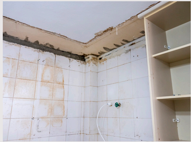
B Steamed up or damp/wet walls
