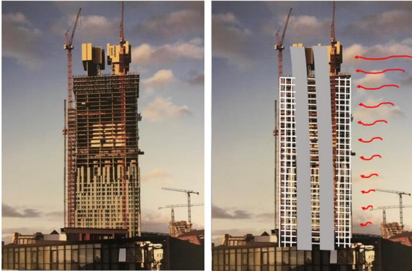
Figure 6.1.13 Beetham tower during construction. Figure also shows, with an animation, how the two cores are assisted by moment frame action to resist lateral wind forces.
