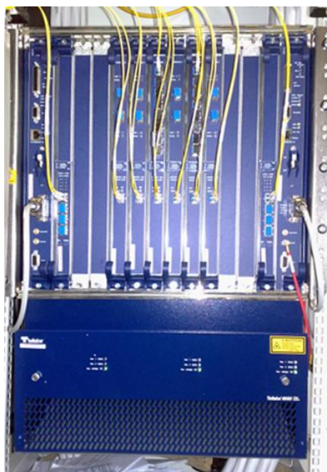
Figure 81: Tellabs 8660 MSSR at TN site
