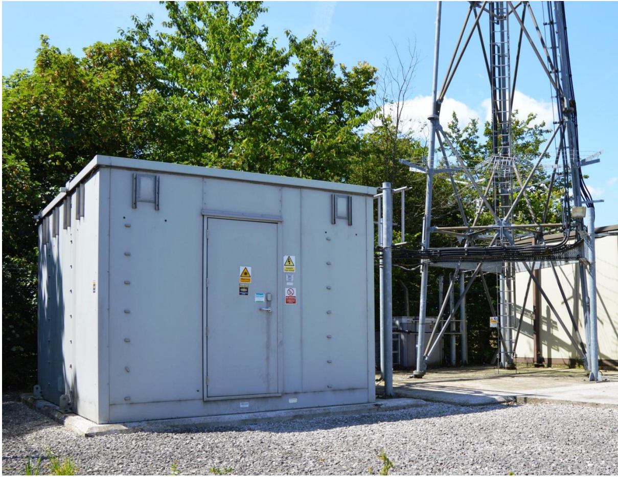
Figure 31: Type 3F Enclosure at site reference CHS0029 in Stretton, Warrington, Cheshire (installed in 2001 and removed in 2017 (photo 2015))
