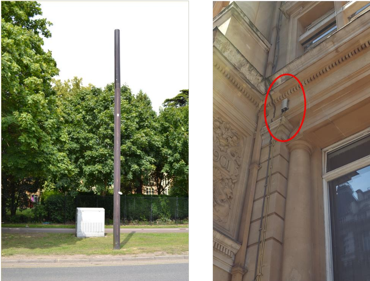
Figure 59: Micro-cell installations examples, street-works (left) (2014) and building mounted (right) (2017)
