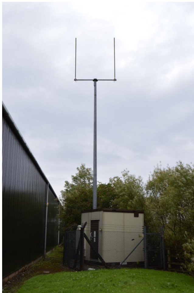
Figure 6: 900 MHz GSM omni-directional cell site (2014)
