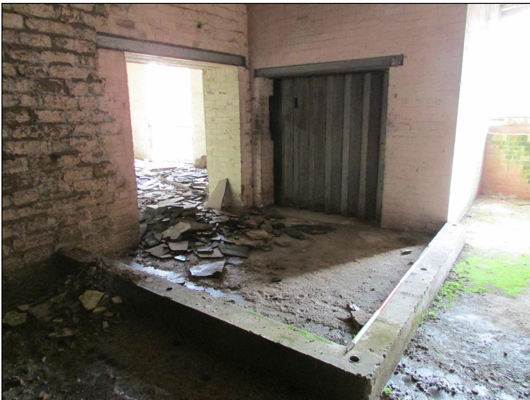
Plate 56 A possible screen around the lift shaft forces movement through the later entrance
