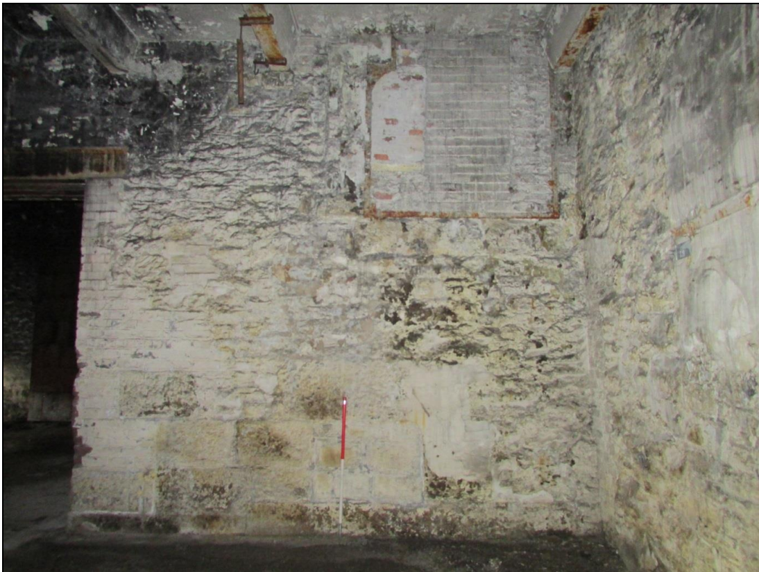
Plate 38 Although plastered over, the dividing wall of the engine house consists of mixed stone coursing types, including random rubble and coursed ashlar blocks. Also shown is a bearing box for the power transmission
