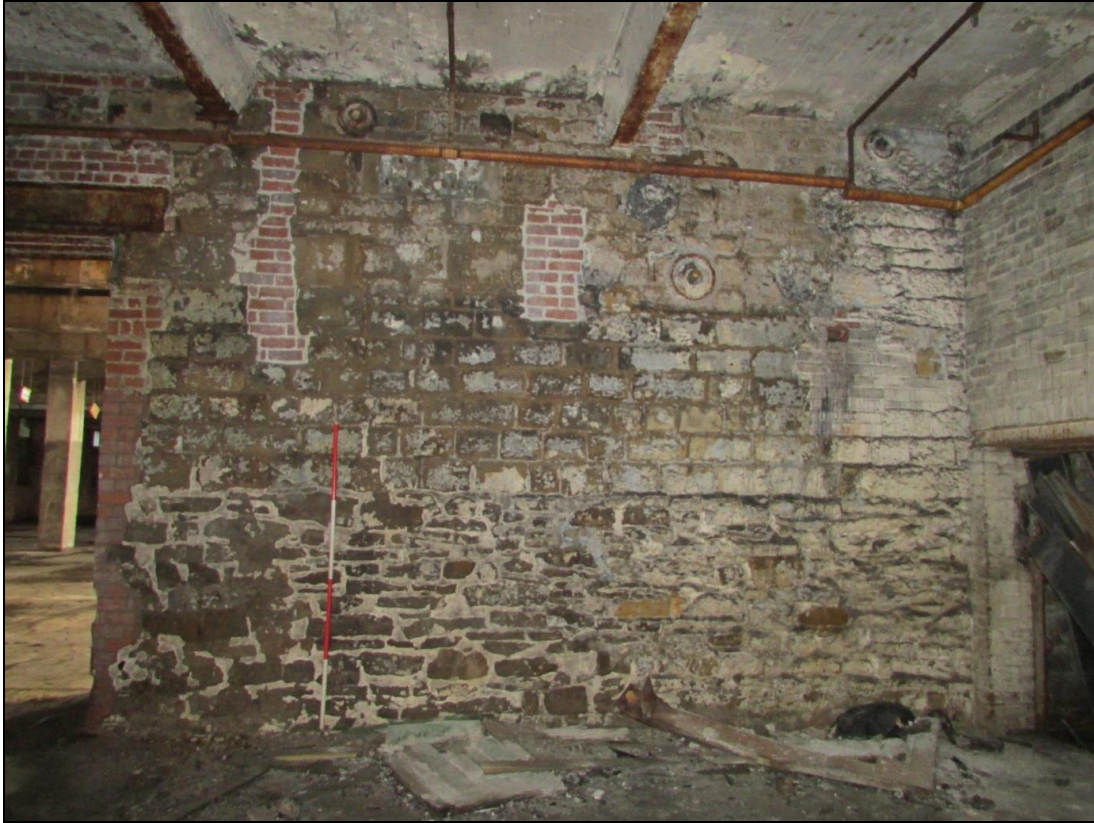
Plate 40 Examples of later brick repairs within the gearing wall, possibly after removal of the engine
