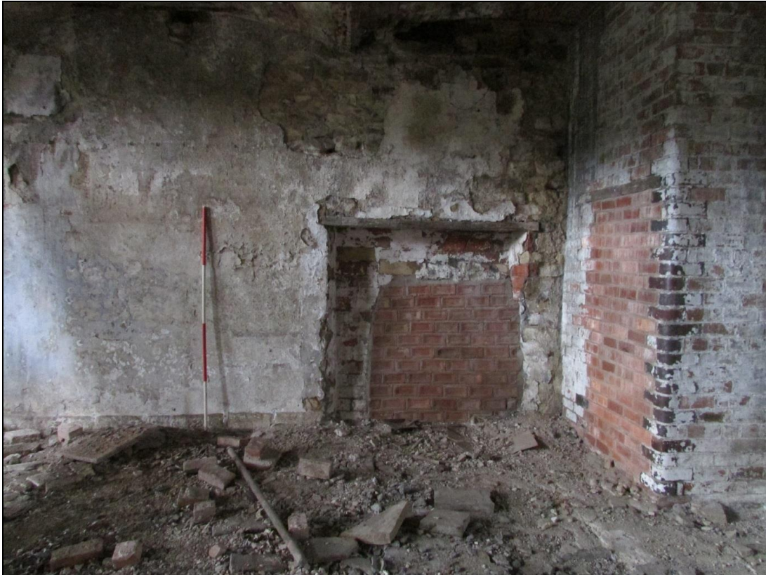
Plate 61 Blocked recess on the third-floor of the engine house. To the right is the blocked entrance into the void
