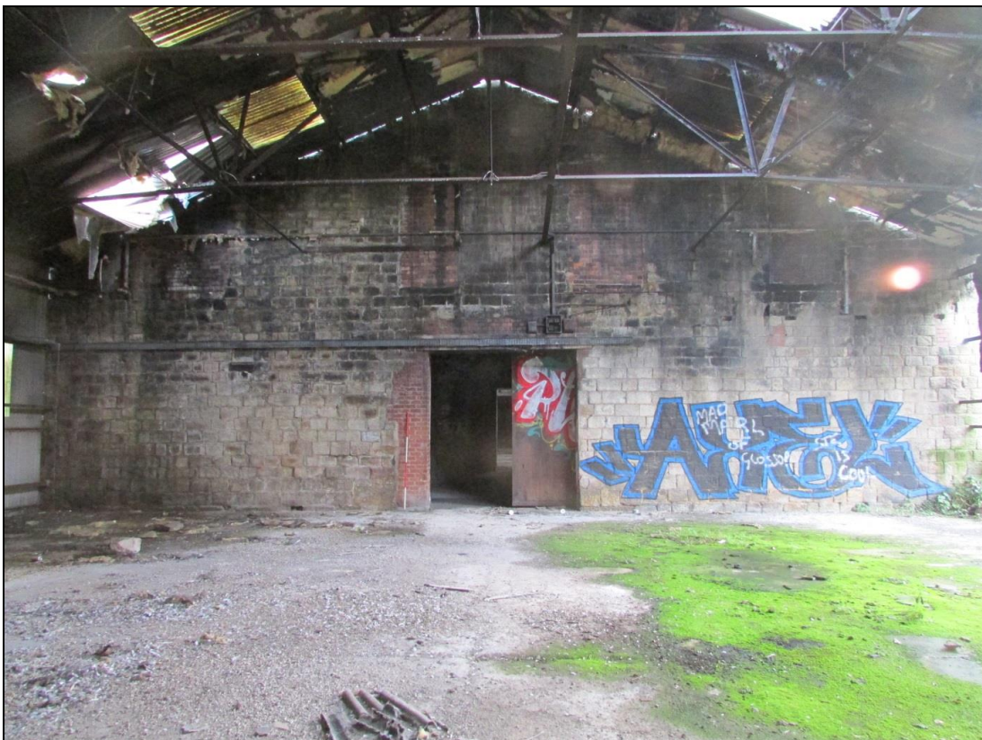
Plate 33 Close up of inserted ground floor entrance and blocked entrances on the first-floor
