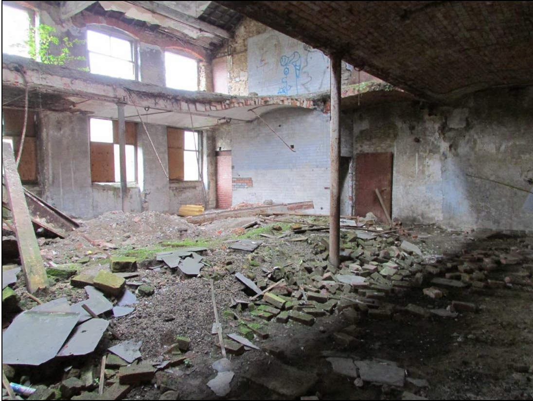
Plate 59 Ceiling collapse on the third-floor of the engine house
