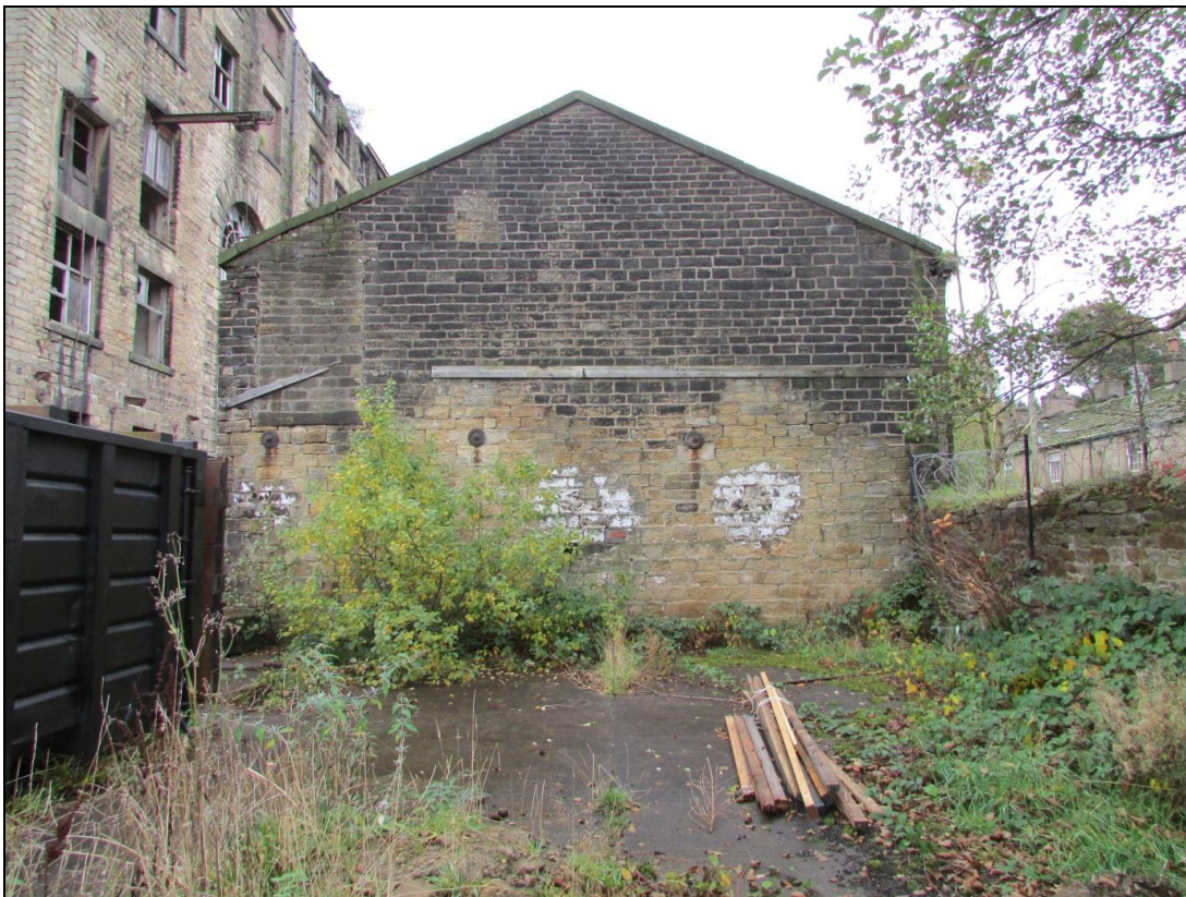
Plate 85 Western elevation of the west shed. A blocked entrance/window can be seen in the top left corner as well as the outline of where another shed abutted
