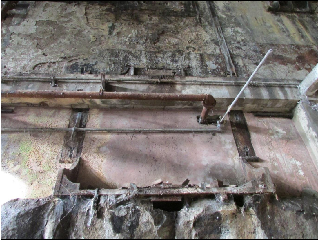
Plate 12 Close-up of the footstep bearing for the driveshaft
