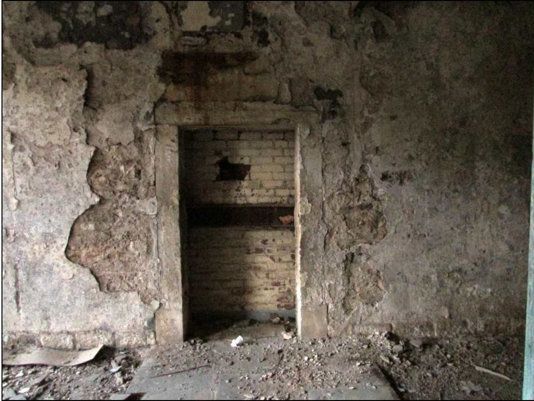
Plate 50 Blocked entrance which would have connected the engine house with the other spinning mill
