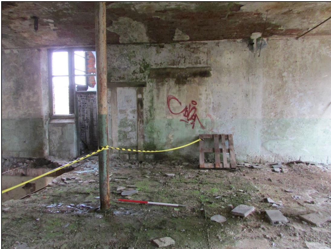
Plate 25 The later entrance to the privy tower extension is evident to the left, with two former entrances blocked to the right
