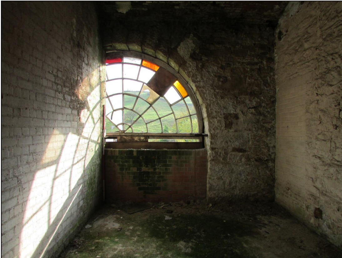
Plate 55 The original fanlight of the engine house was blocked by the lift shaft (to the left) and a c.1.00m high brick partition
