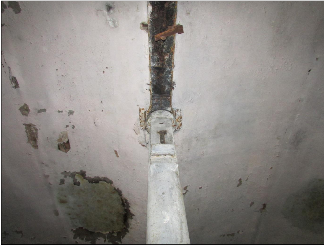
Plate 8 Close up of a column with a bolting face, supporting the line shaft
