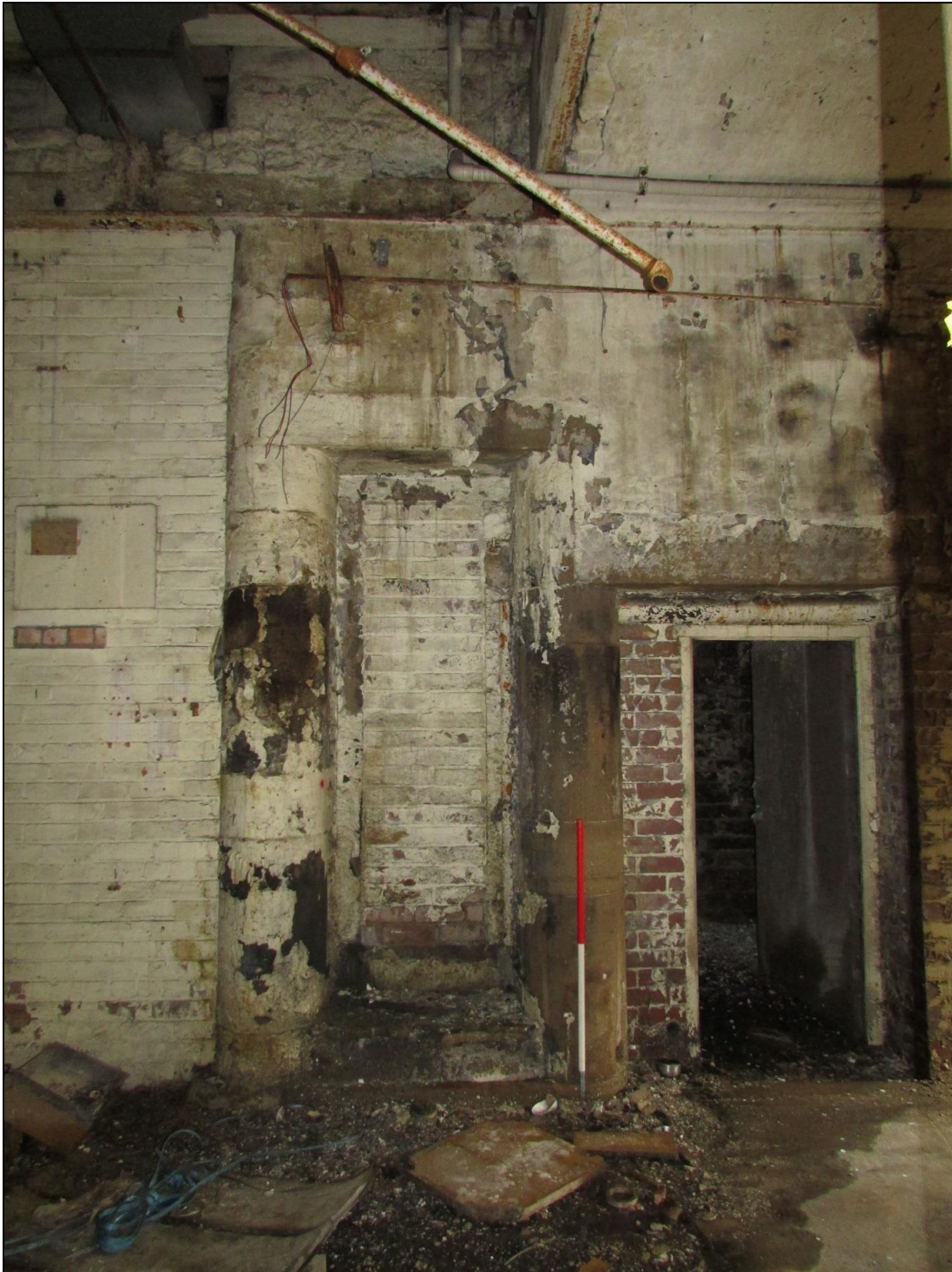
Plate 10 Blocked entrance into the former privy tower, with the later entrance to the lift shaft on the right, subsequently made smaller
