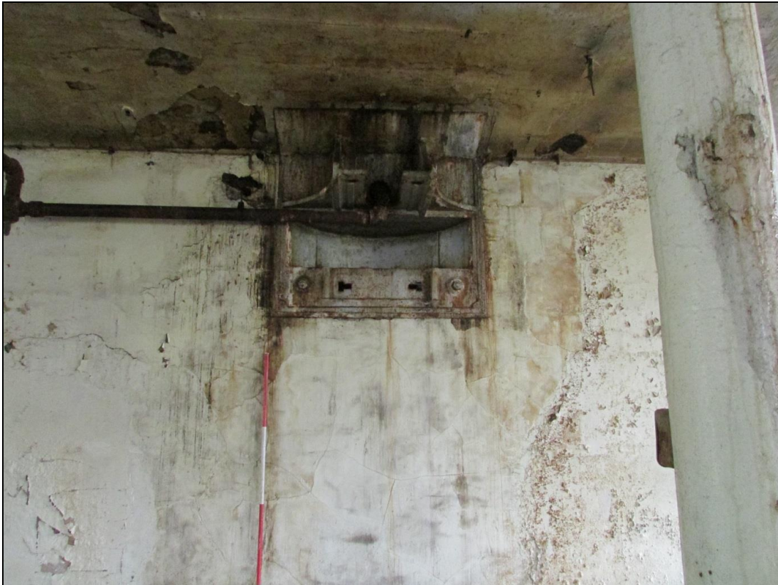
Plate 22 Metal bracket on the second-floor gearing wall to support the upright shaft
