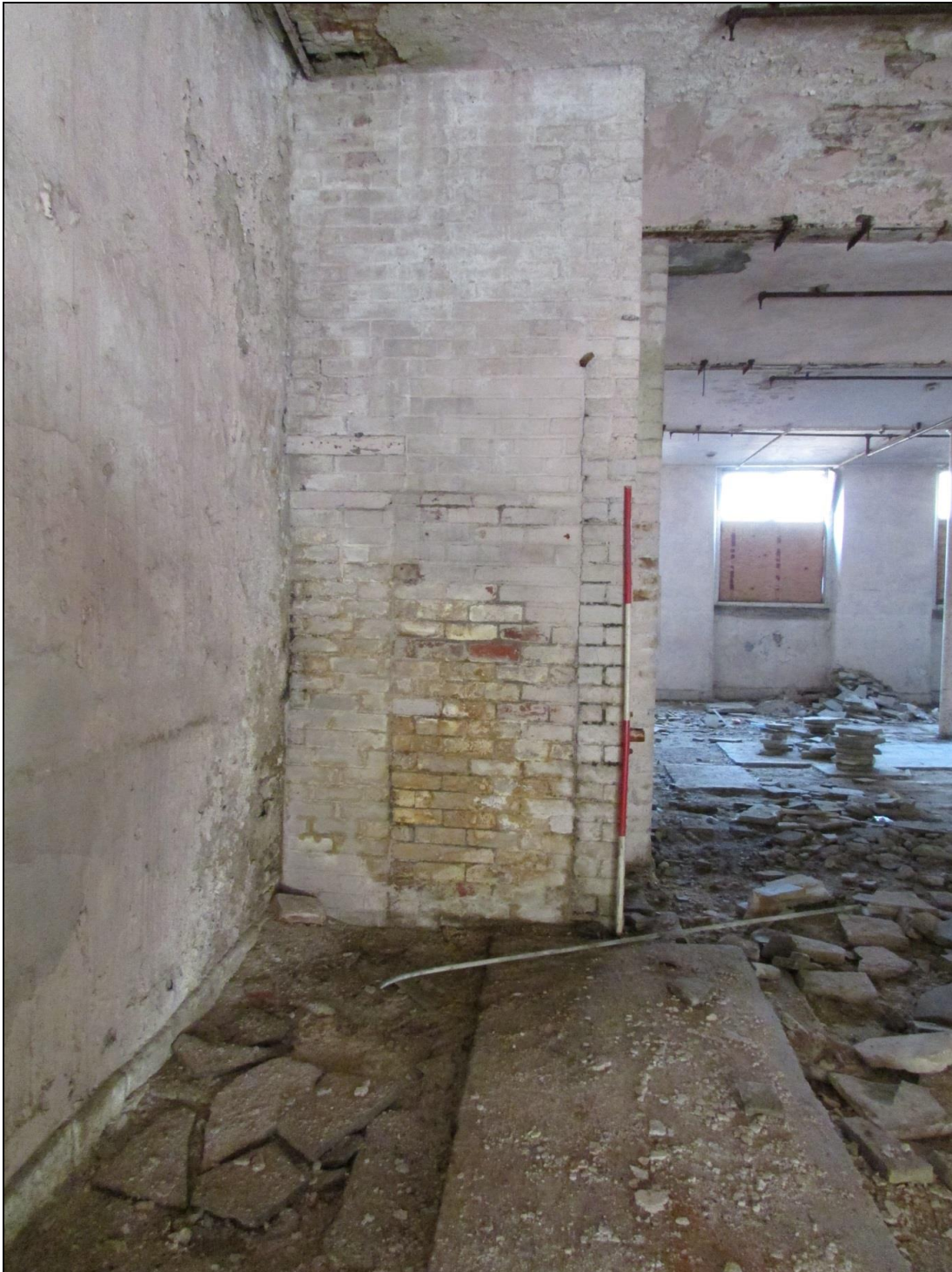
Plate 52 Blocked entrance into a later sub-division, creating a void behind which could not be accessed
