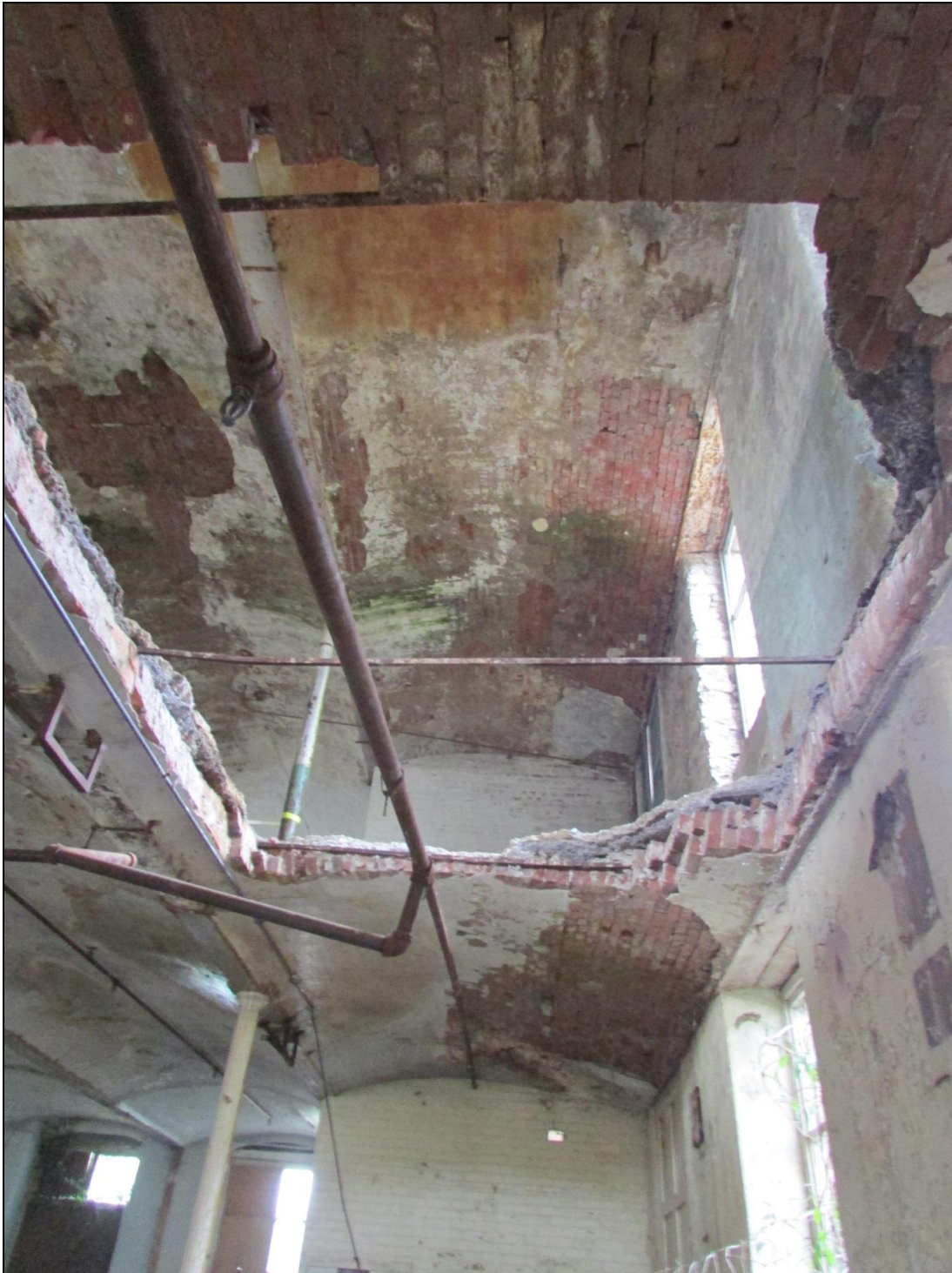
Plate 17 A small part of the second-floor ceiling had collapsed within the eastern part of the mill, exposing the metal tie-beams integral to the fireproof arches' structure
