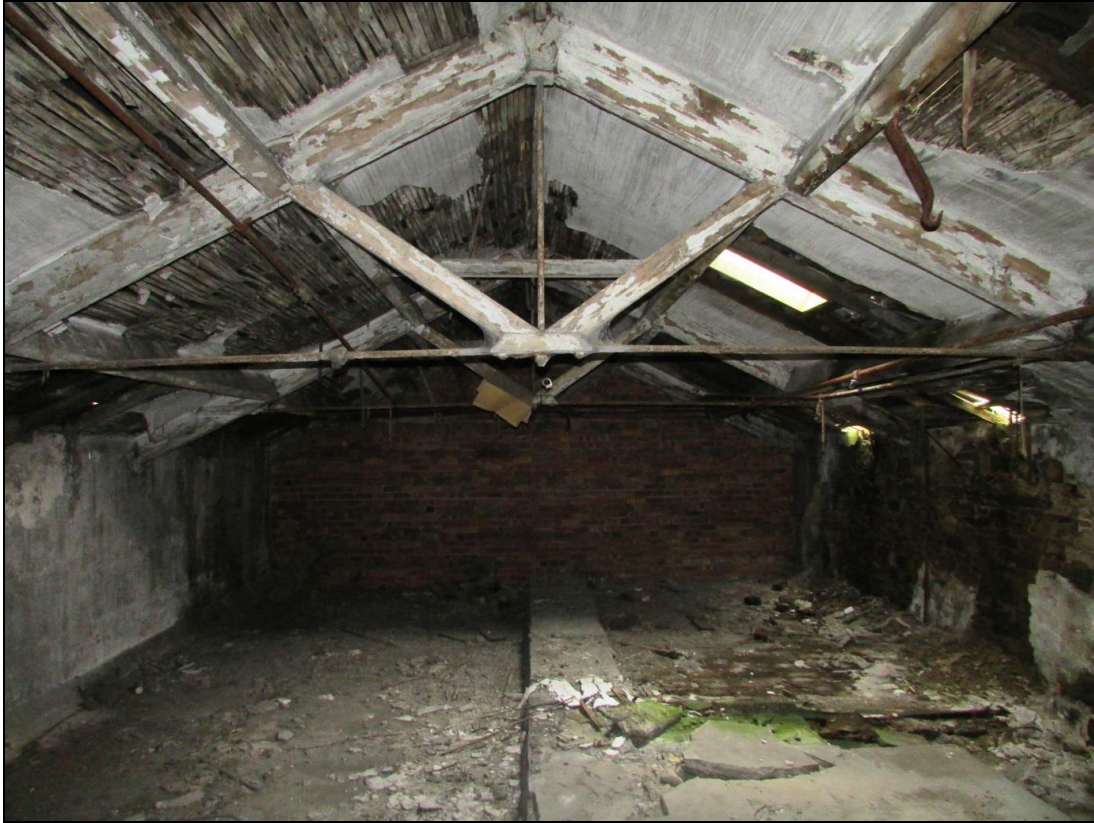
Plate 75 Office Block third-floor. The later southern elevation is visible at the rear, as well as the single span roof incorporating both iron and timber
