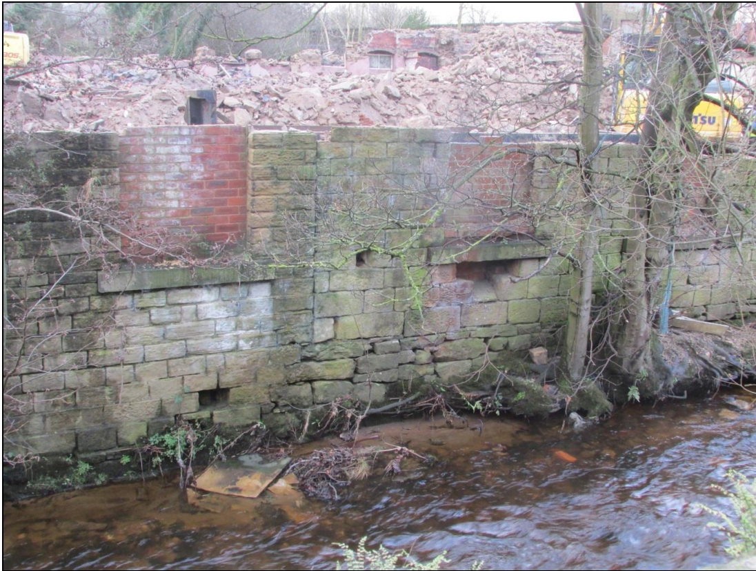
Plate 82 The butt joint between the earlier shed (east) and the later shed (west) is clearly visible, as well as where the later shed partly used the drystone foundations of the earlier building
