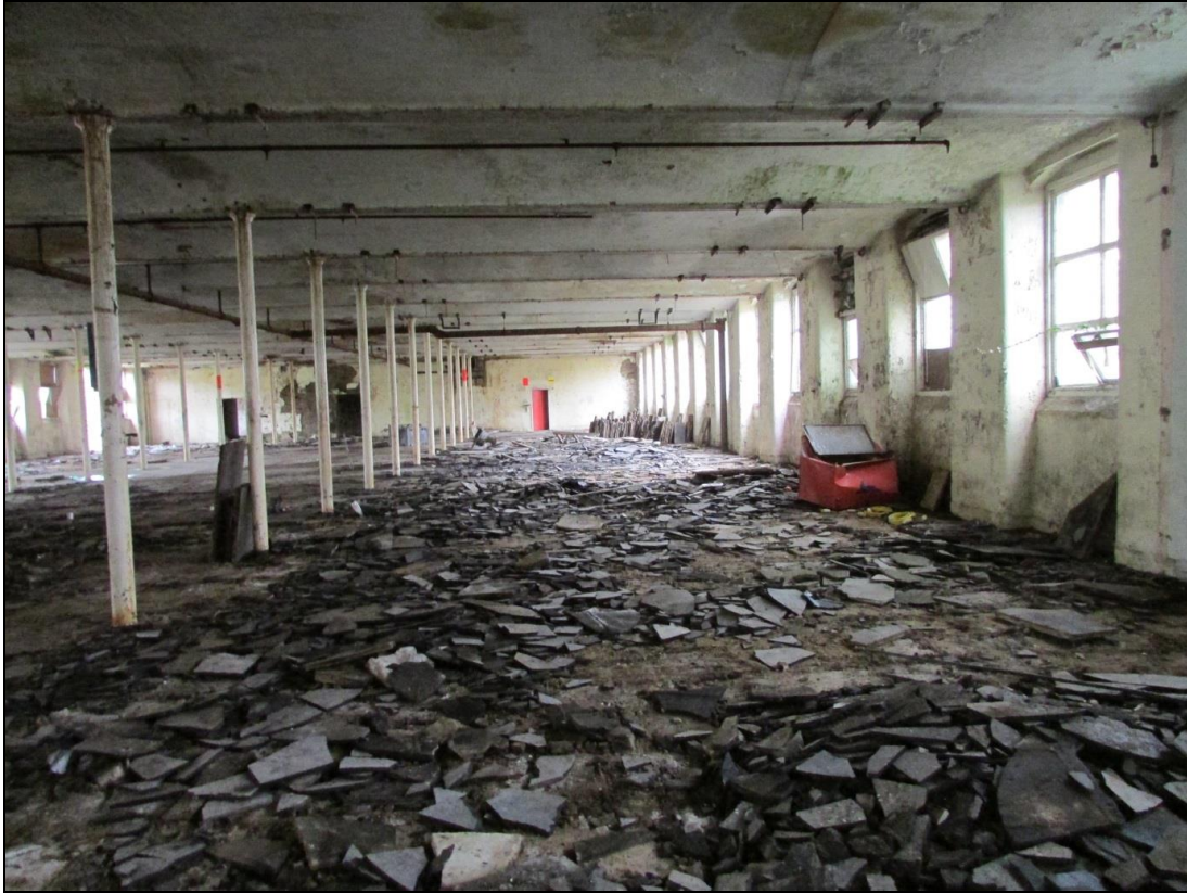
Plate 18 Visible on the beams within the ceiling are two lines of lineshaft hangers, which helped power the machinery
