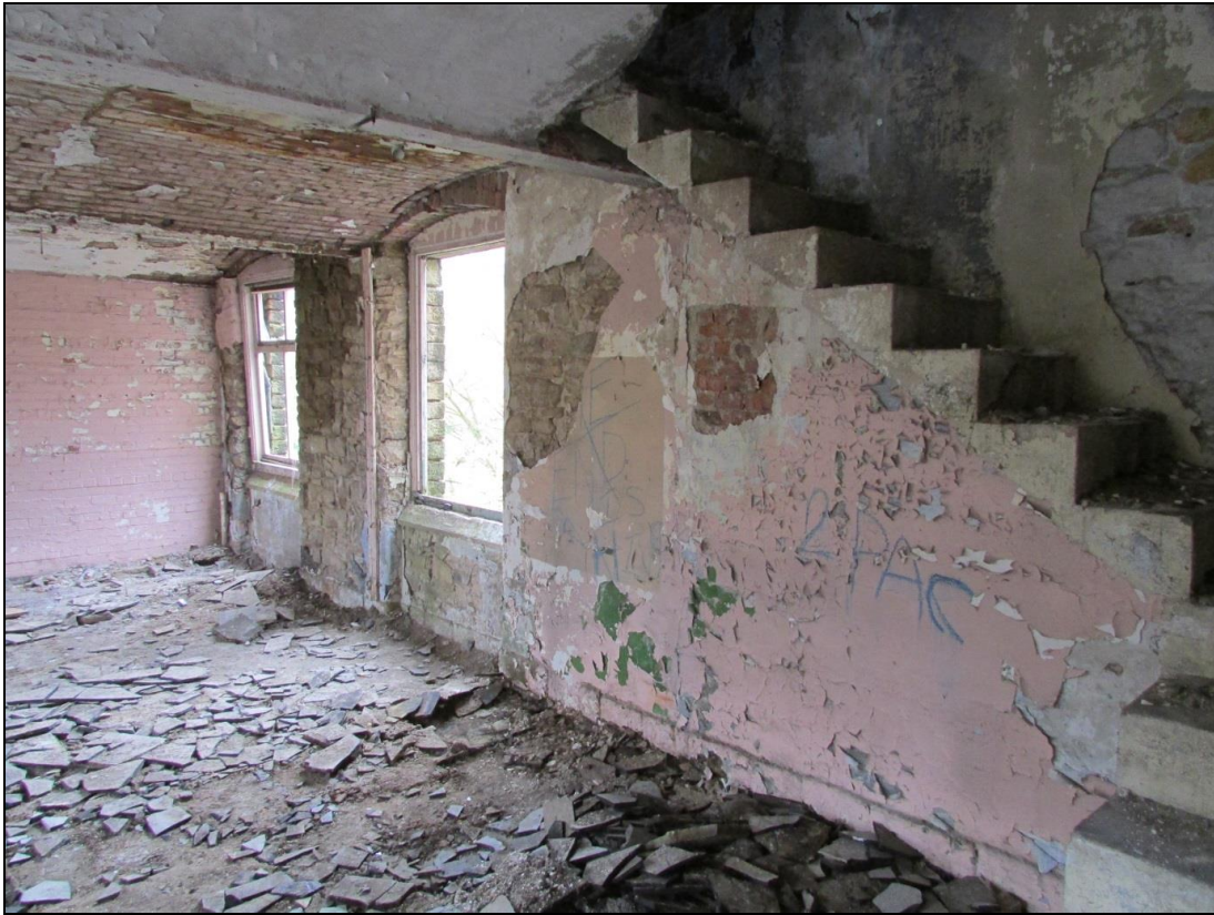
Plate 74 Later steps leading to the third-floor within the office block. Also visible beneath the plaster is the brickwork blocking one of the windows
