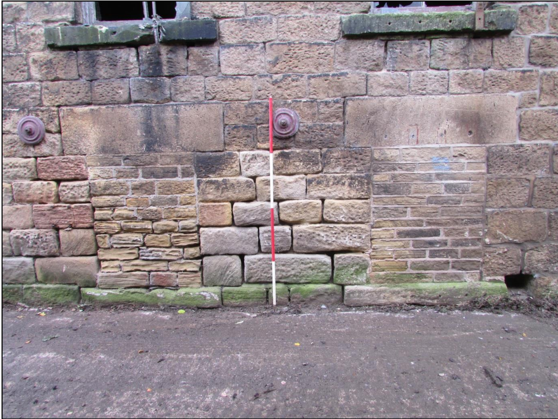
Plate 36 Two former windows blocked up on the ground-floor of the engine house
