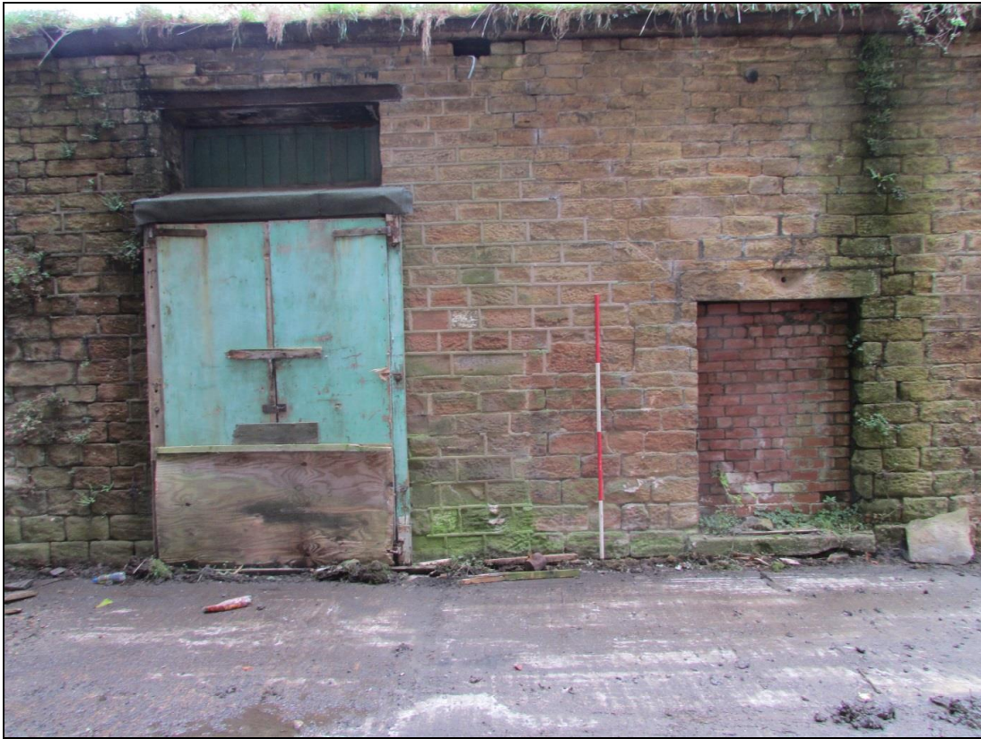
Plate 77 A door was inserted into the northern elevation of the east shed (left) and a window was also blocked at a later stage
