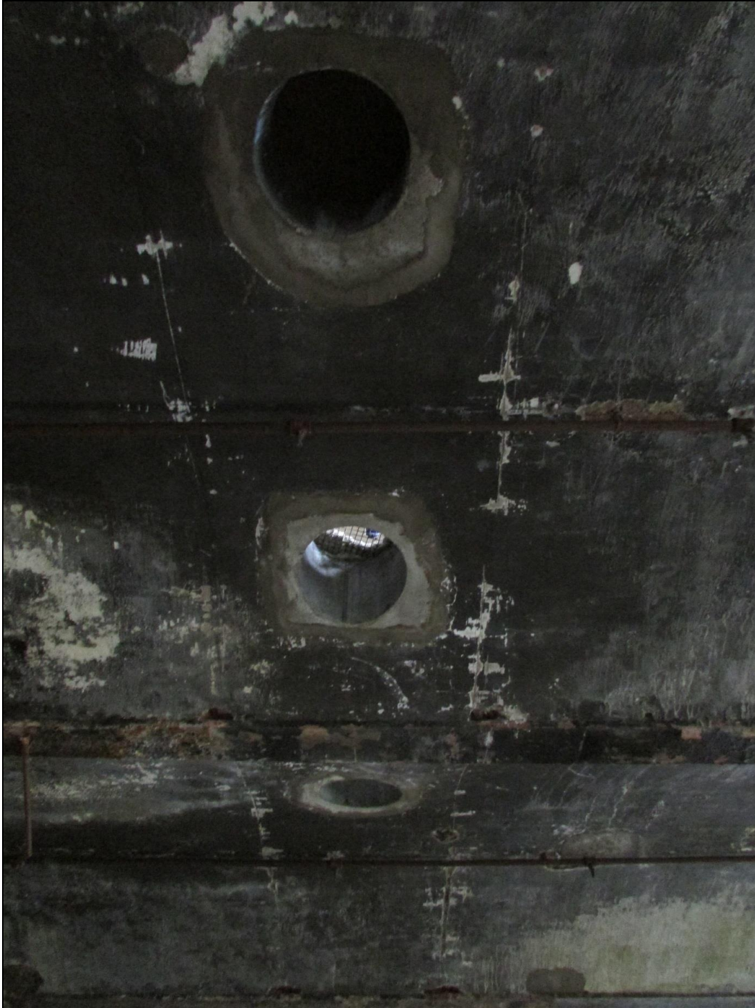
Plate 15 Small circular apertures inserted at a later date into the first-floor ceiling
