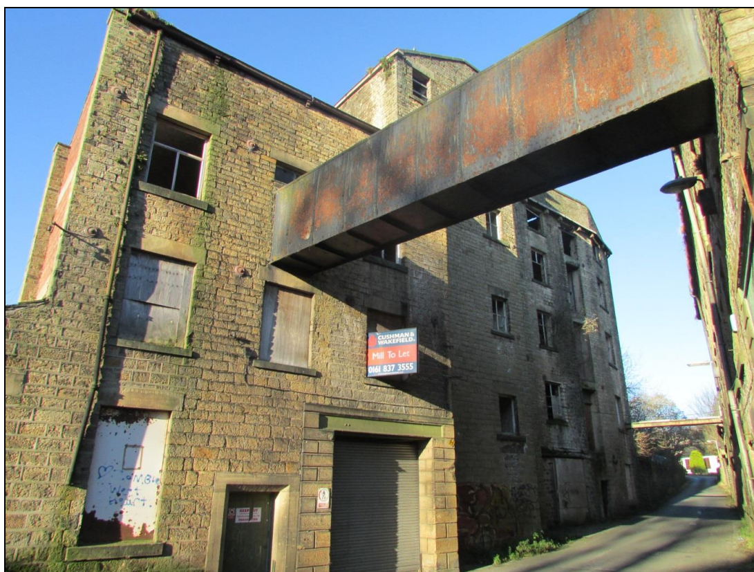
Plate 64 Eastern elevation of the office block, with the later metal walkway visible (access was not possible during the survey – this photo dates to December 2014)
