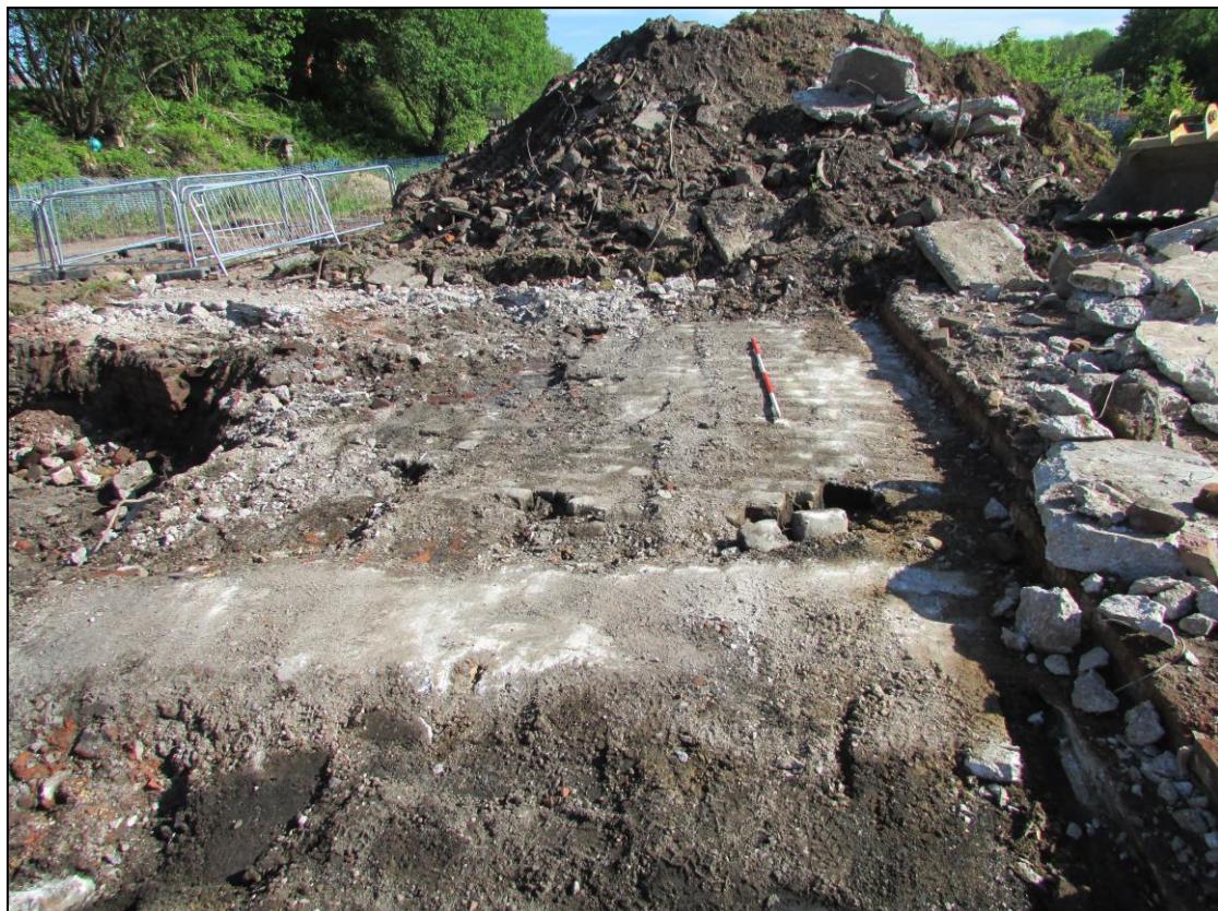
Fig. 41. Northern side of watching brief area showing an extension of the concrete floor revealed during the 2014 evaluation. Looking north.
