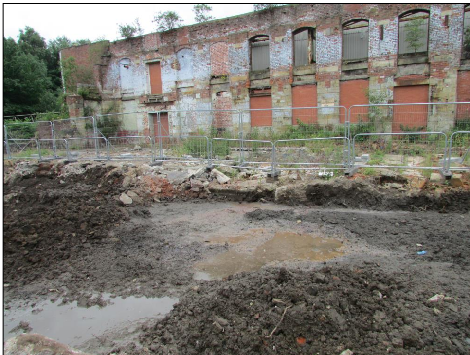
Fig. 18. Area of watching brief showing the lack of features below the concrete raft floor of the 20 th century mill structure.
