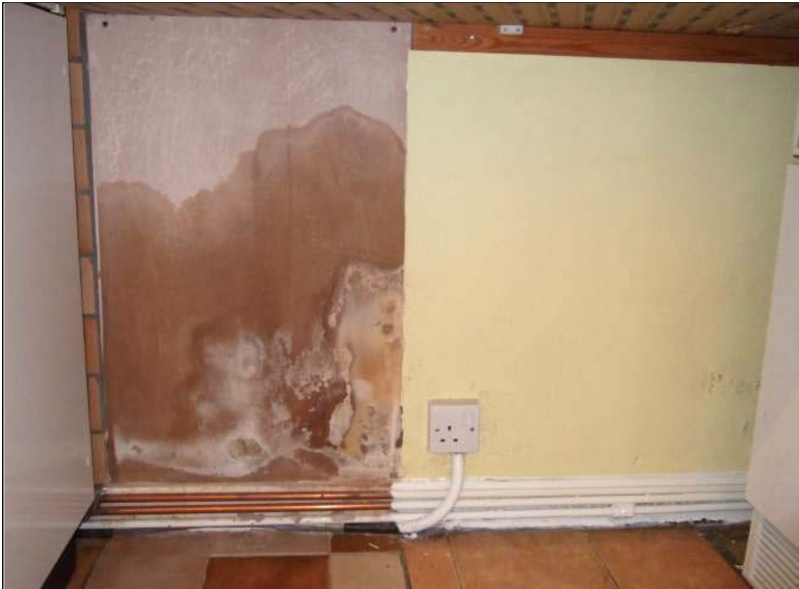
Figure 10: Wall base dampness aligning with the Sharp Front model (example 3).
