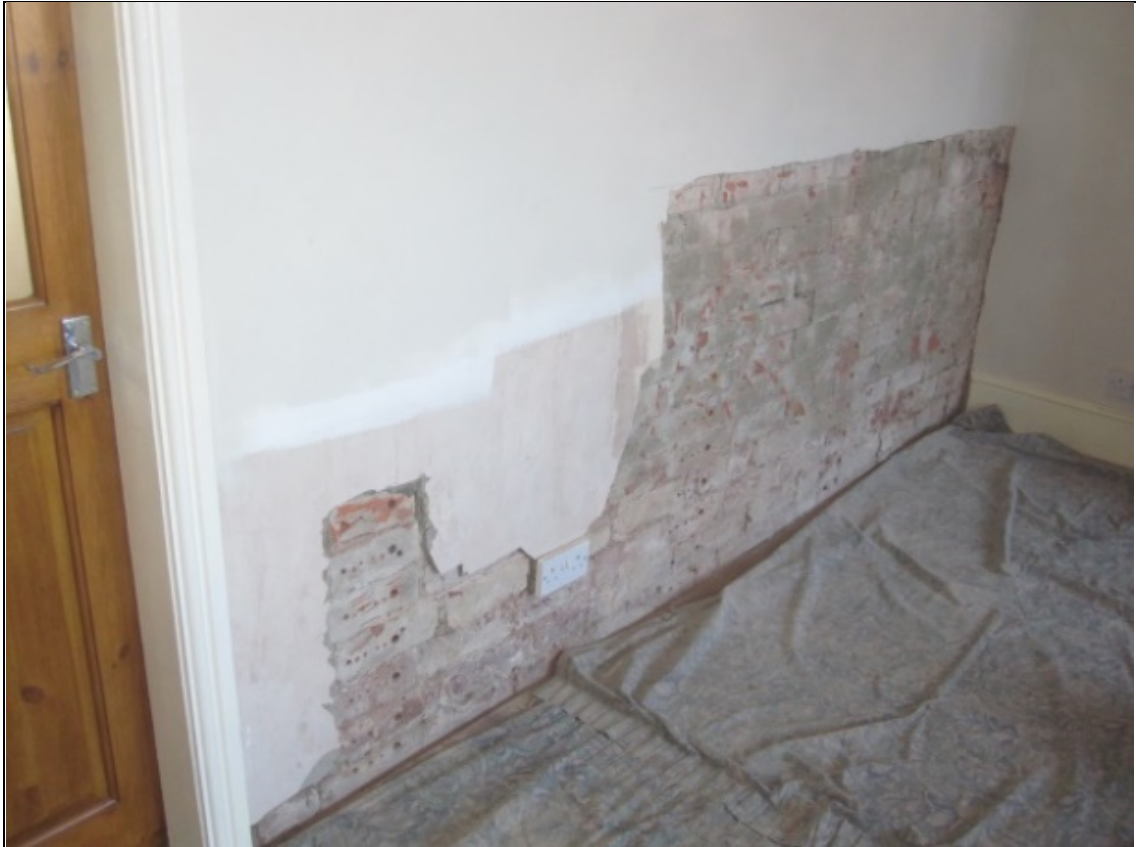
Figure 108: Test Panels C, D, and E with plasterwork removed to facilitate masonry sampling.
