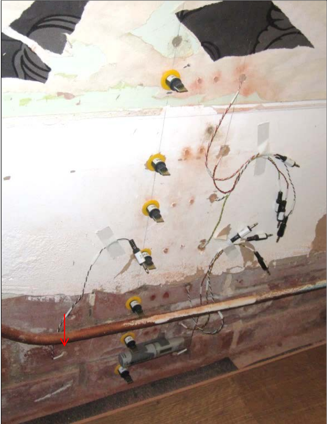
Figure 84: Panel A with additional Timber Probe Type 1 installed in row 2.
