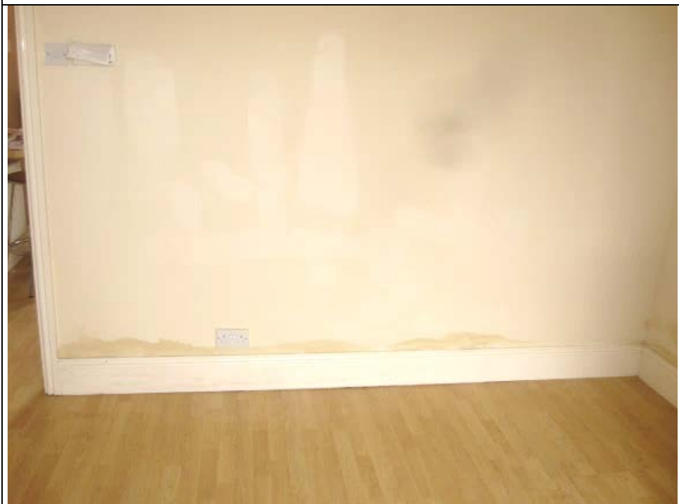
Figure 17: Living room rear wall. Damp staining extends to 250 mm above floor level.
