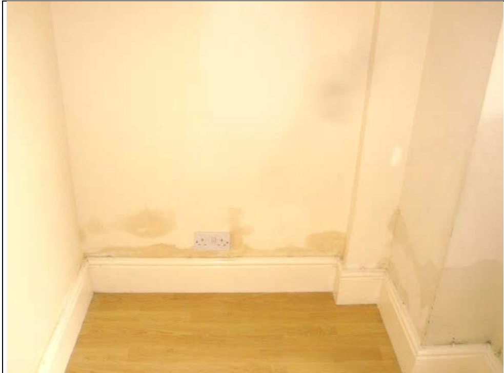
Figure 18: Living room right-hand side (party) wall; rear alcove. Damp staining extends to 400 mm above floor level.
