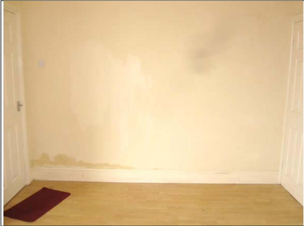
Figure 16: Living room left-hand side (party) wall. Damp staining extends to 300 mm above floor level.
