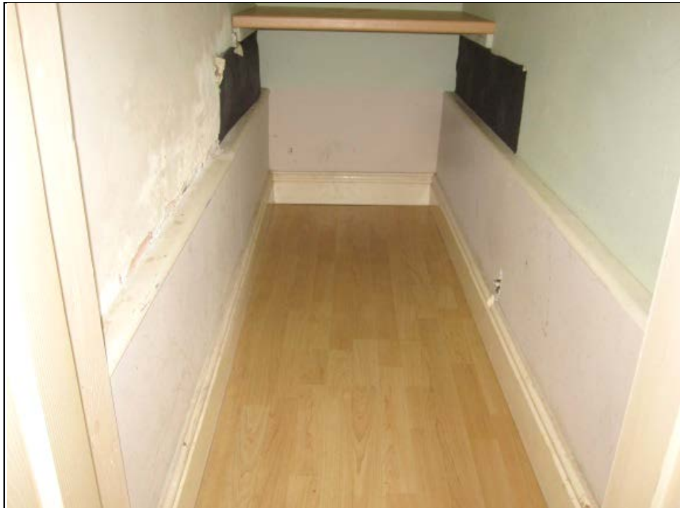
Figure 22: Understairs cupboard left-hand side and right-hand side walls. Damp staining extends to 800 mm above floor level.
