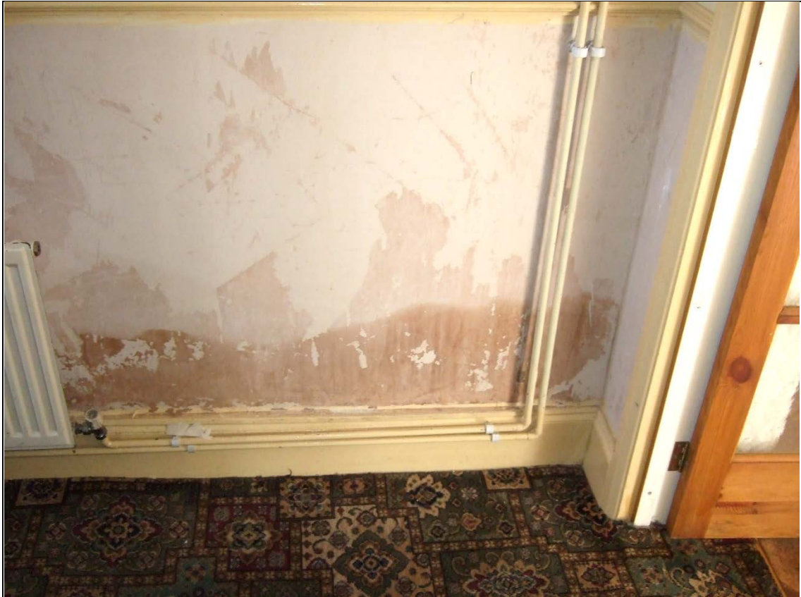
Figure 9: Wall base dampness aligning with the Sharp Front model (example 2).
