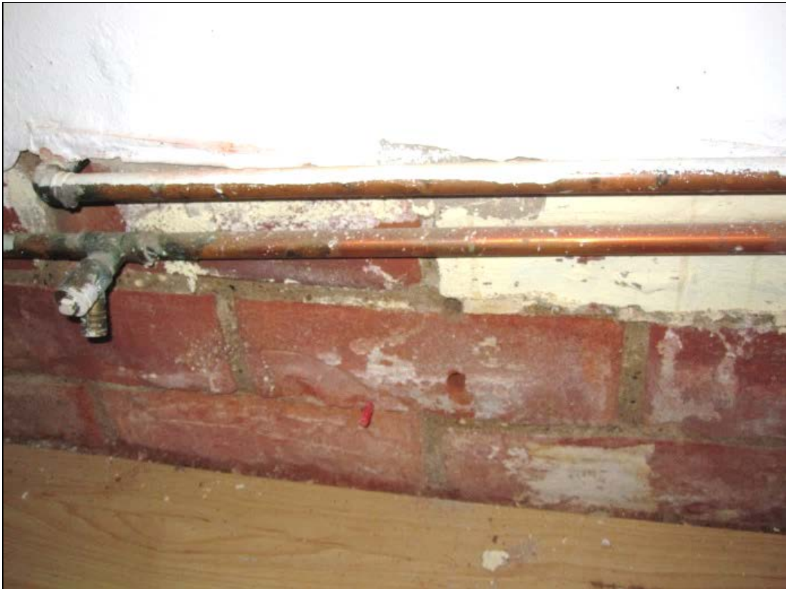
Figure 59: Understairs cupboard removal of samples from Panel A for Stage 1 moisture analysis.
