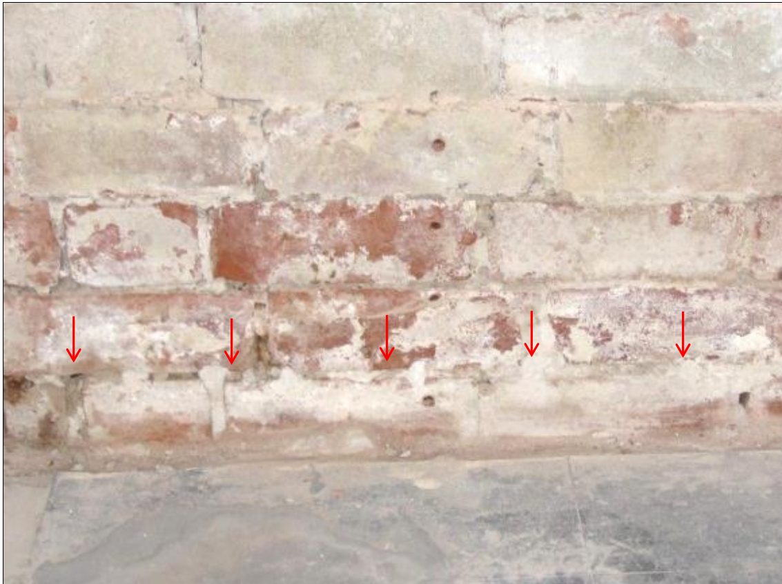
Figure 25: Living room rear wall evidence of chemical injection damp proof course.
