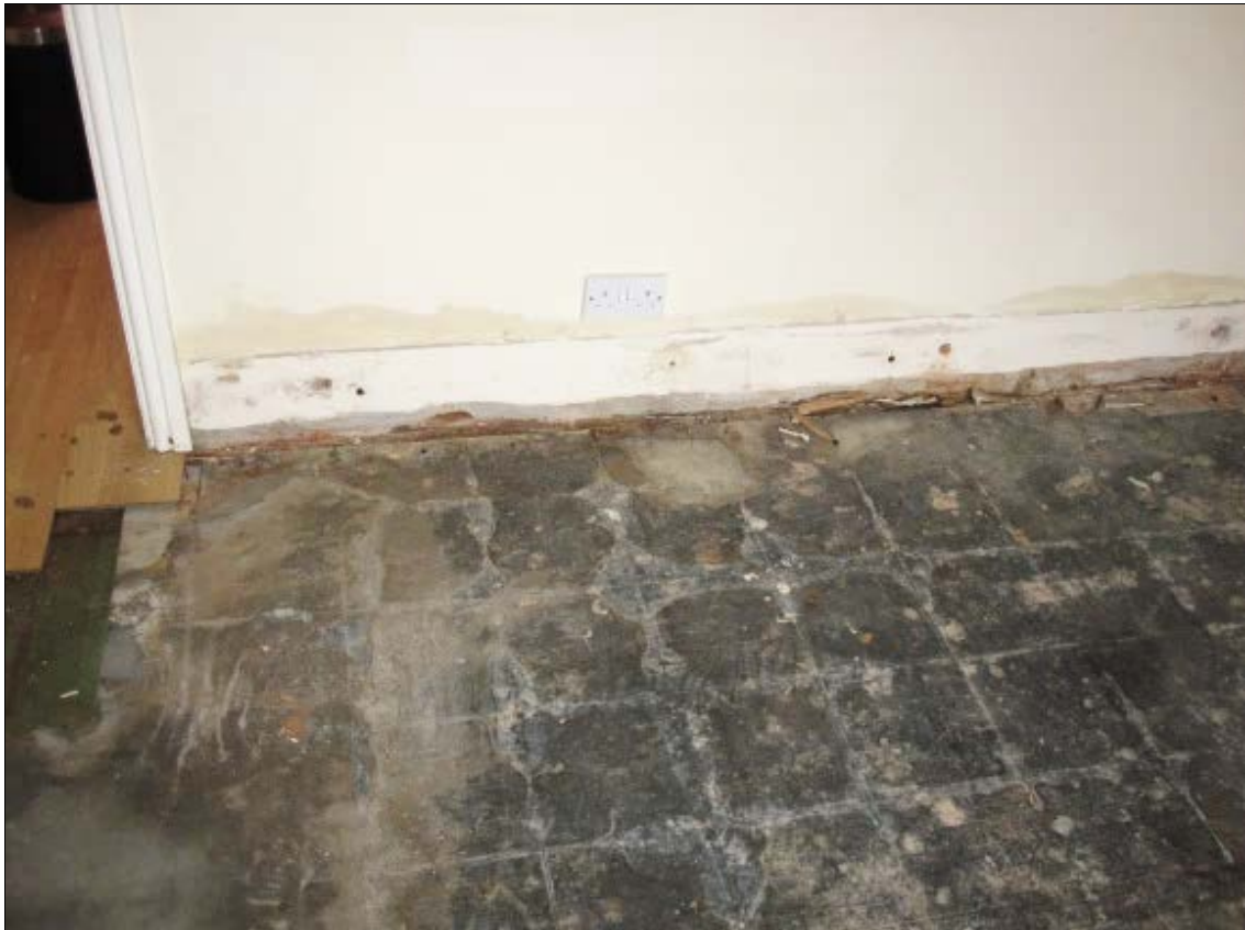
Figure 33: Base of the living room rear wall: plaster bridges the existing chemical injection damp proof course.
