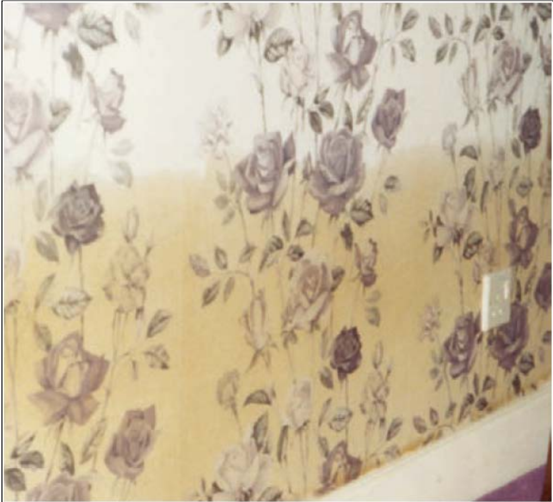
Figure 4: Staining to wall paper on a wall affected by rising damp (Adapted from Trotman, 2007, p. 1).
