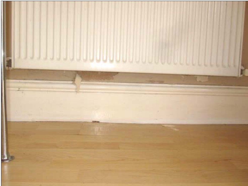
Figure 20: Kitchen left-hand side wall. Damp staining extends to 350 mm above floor level.
