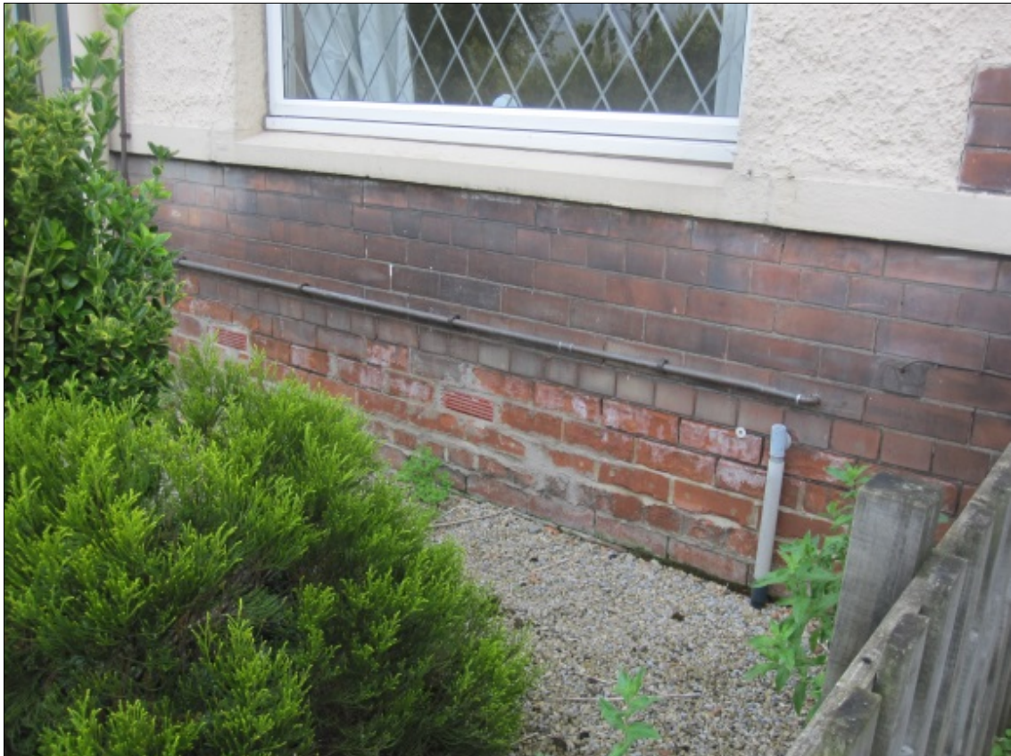
Figure 30: Front wall perished masonry.
