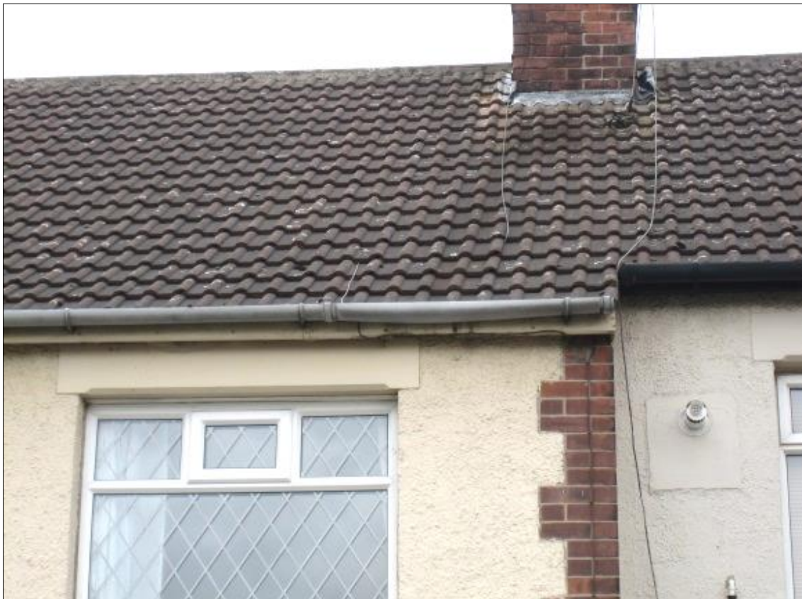
Figure 28: Gutter above right-hand end of front elevation.
