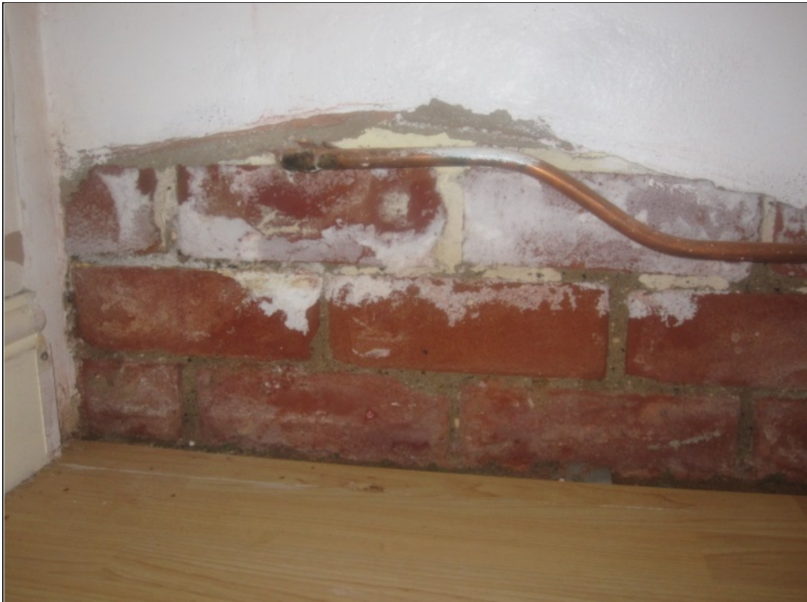
Figure 57: Understairs cupboard right-hand side wall (location of Panel A) illustrating the construction found behind the dry lining.
