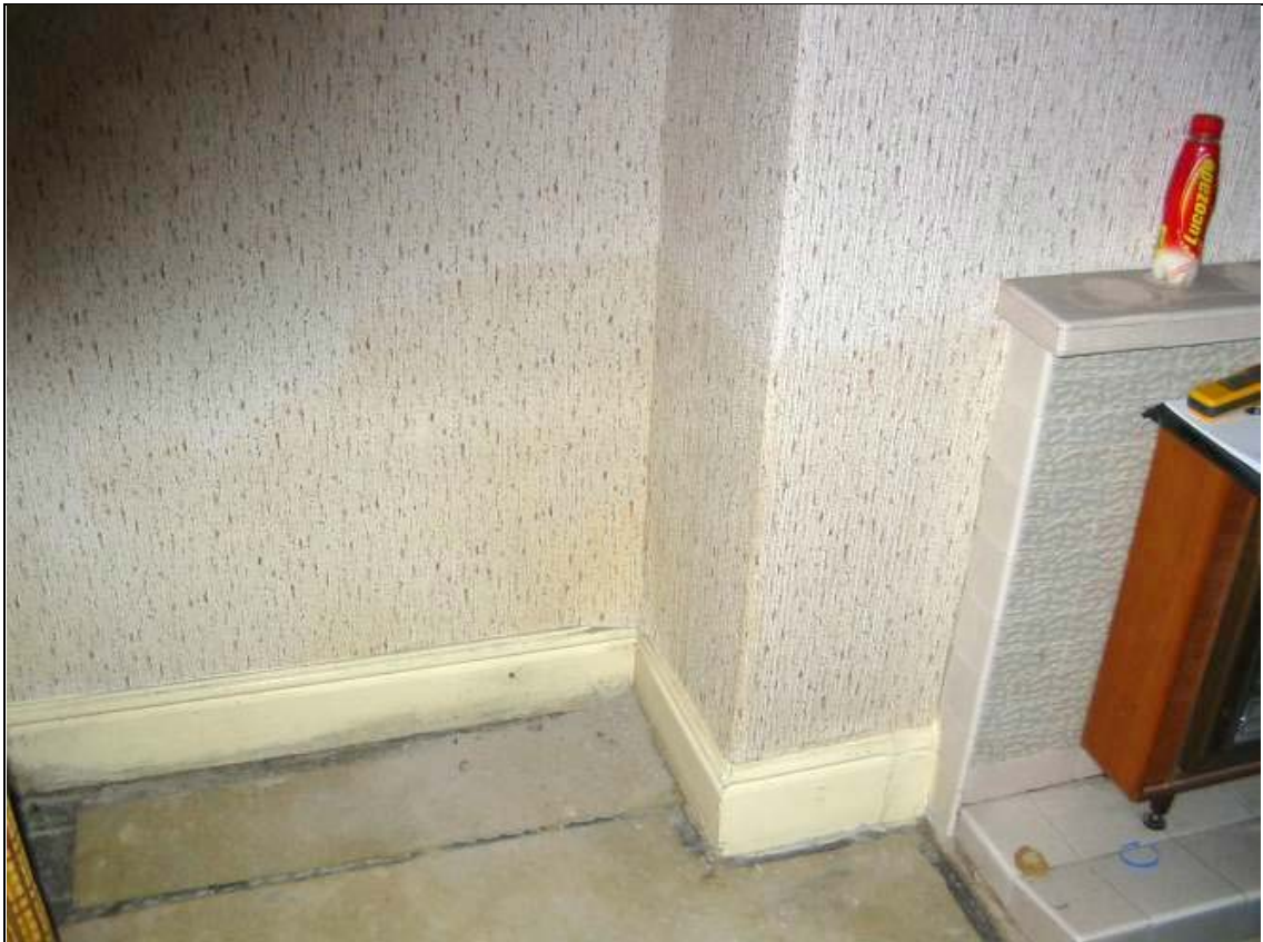
Figure 8: Wall base dampness aligning with the Sharp Front model (example 1).
