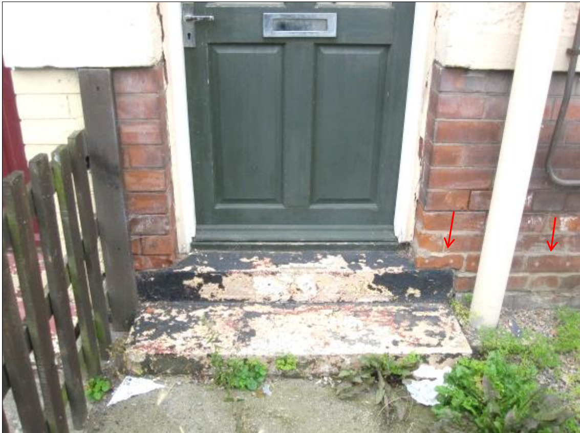
Figure 24: Front wall evidence of chemical injection damp proof course.
