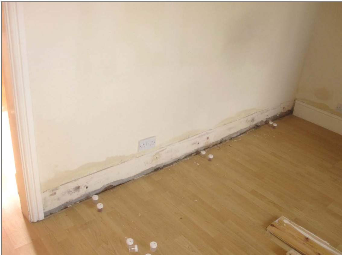
Figure 58: Living room rear wall removal of samples from panel positions C, D, and E for Stage 1 moisture analysis.
