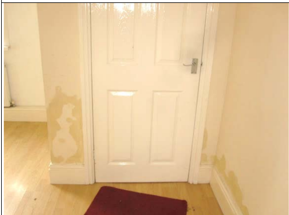
Figure 15: Living room dividing wall with entrance lobby. Damp staining extends to 800 mm above floor level.
