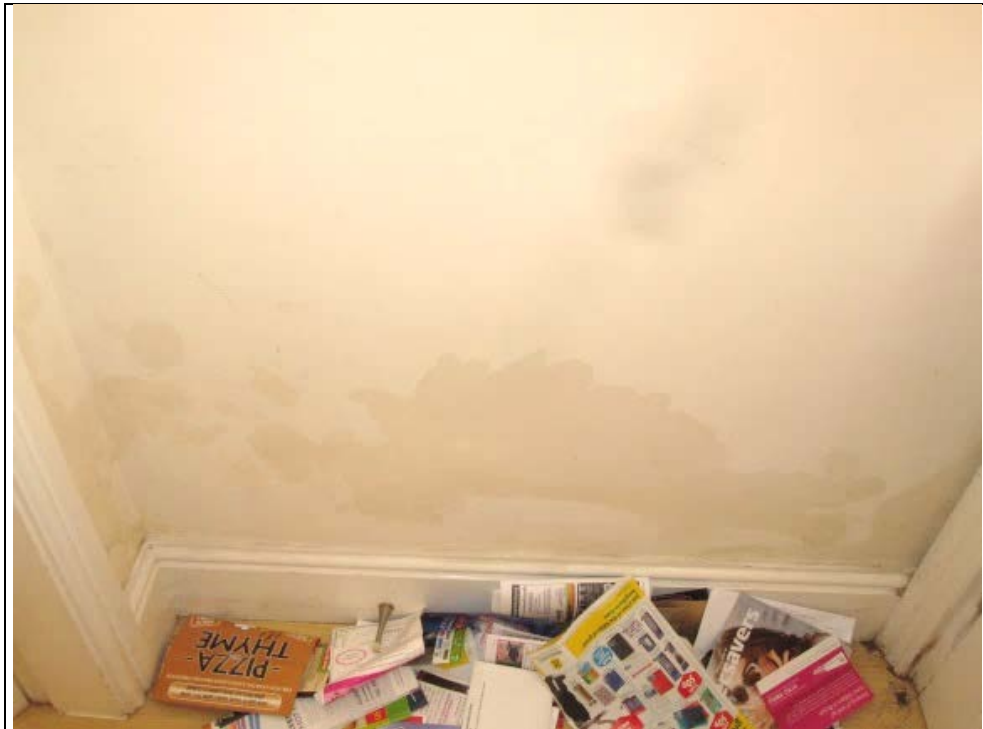
Figure 14: Entrance lobby right-hand side wall. Damp staining extends to 550 mm above floor level.
