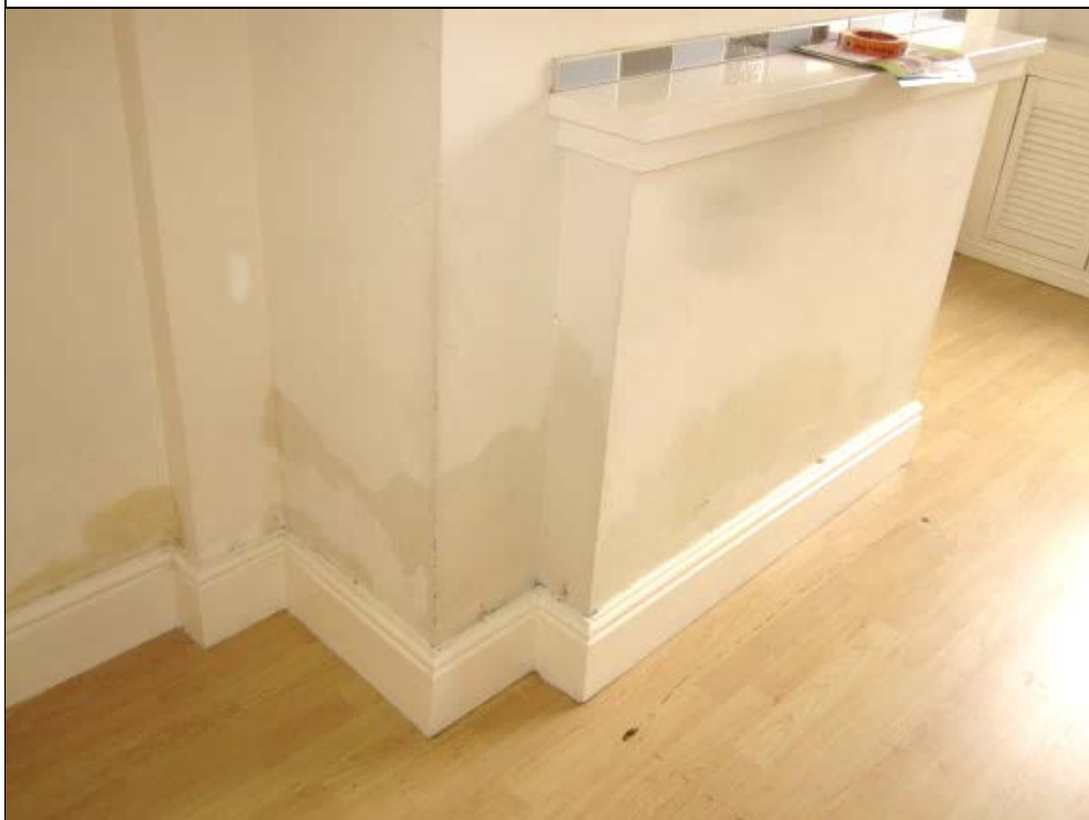
Figure 19: Living room right-hand side (party) wall; fireplace. Damp staining extends to 650 mm above floor level.
