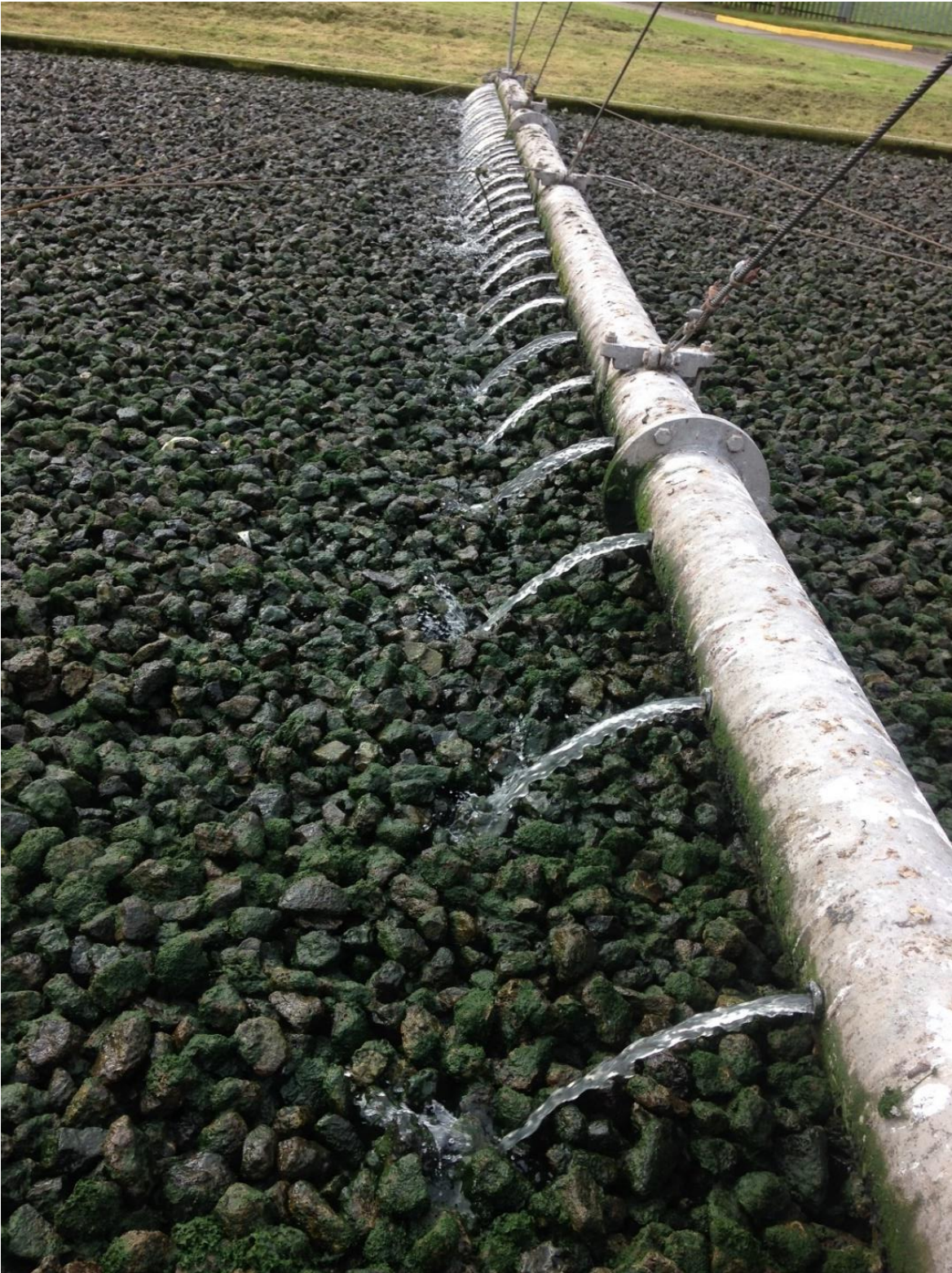
Fig. 3: Influent being dispensed onto the filter bed. Shown is a portion of a filter bed and part of the four-arm rotary distributor covered with bird droppings. The green colour is filter flora - part of the biological film. (Picture by: S. Wenjere).
