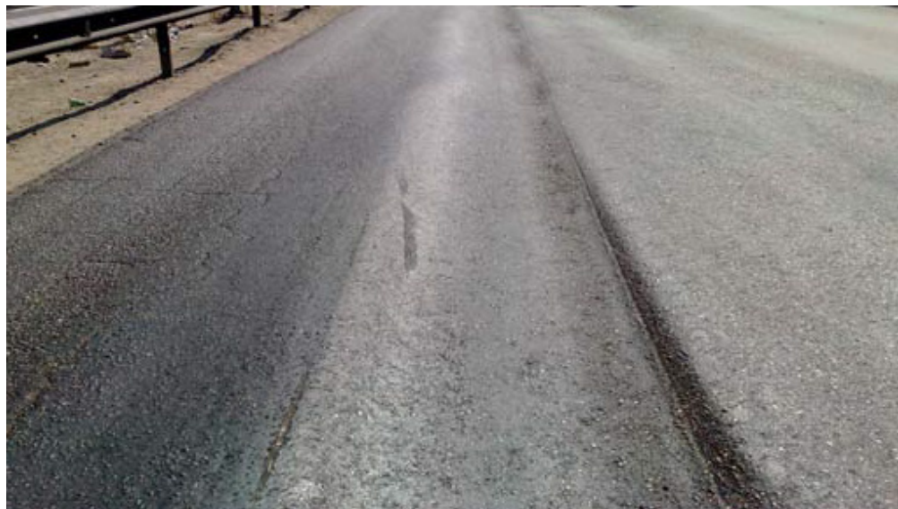
Figure (2-12) Permanent Deformation (Rutting) in Flexible Pavement
