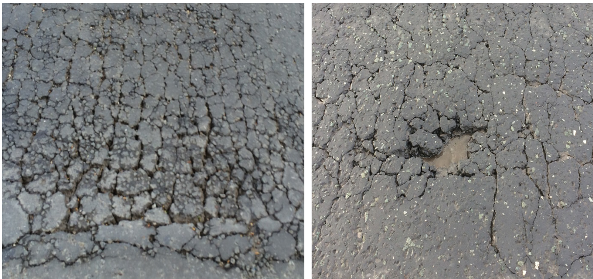
a) Fatigue (Alligator) cracks
