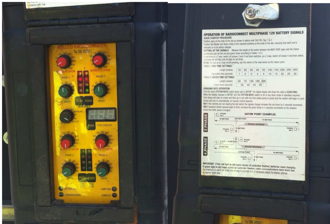
Figure A.38: Photo of the signal control box for temporary traffic signal
