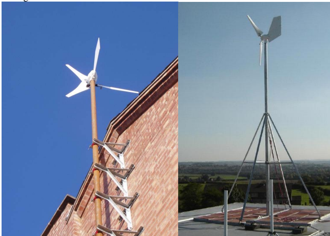
Figure 1: Examples of wall-mounted and roof-mounted installations (photo: Encraft Ltd.)
