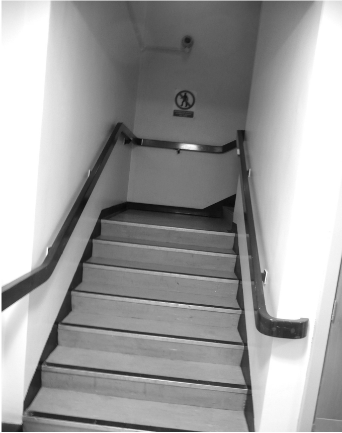
Fig 5. Stairs with 'No Entry' sign
