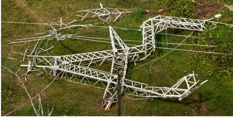
Figure 1-2: A power transmission tower felled by Hurricane Maria (Gallucci, 2018)
