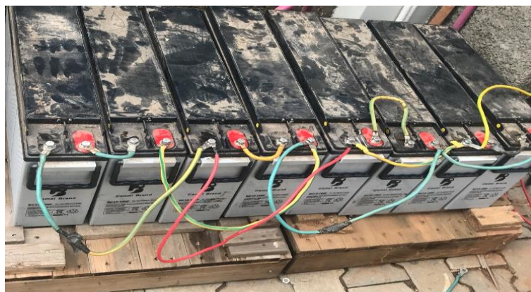
Figure 4:14 Type of the installed GSWHP battery storage
