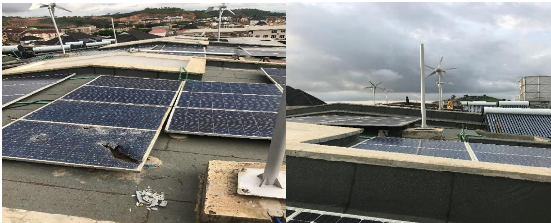
Figure 4:12 Broken solar panels and wind towers.
