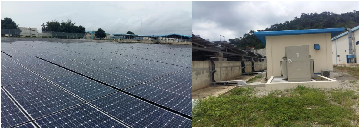
Figure 4:7 Grid-tied solar system connected with the Transformer
